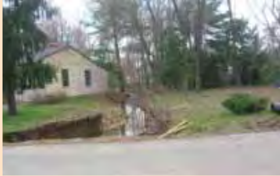
North Fork Accotink Creek bank erosion at Orchard Street
