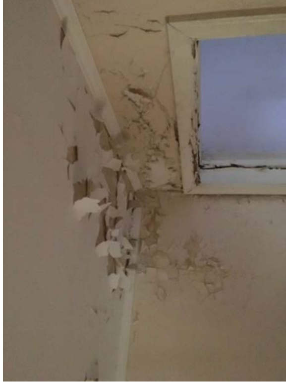
Peeling paint typical throughout building.
