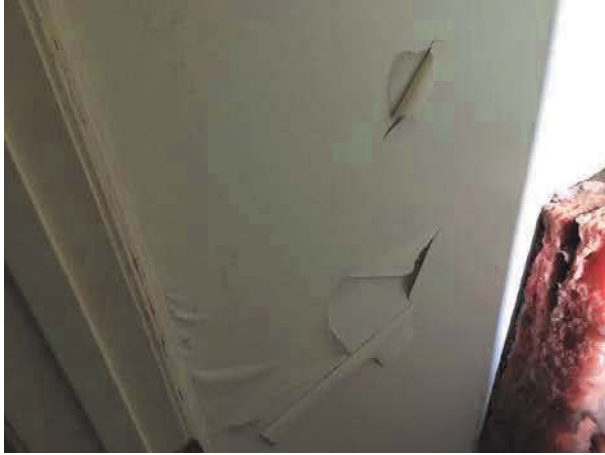
Paint peeling from wall in laundry room
