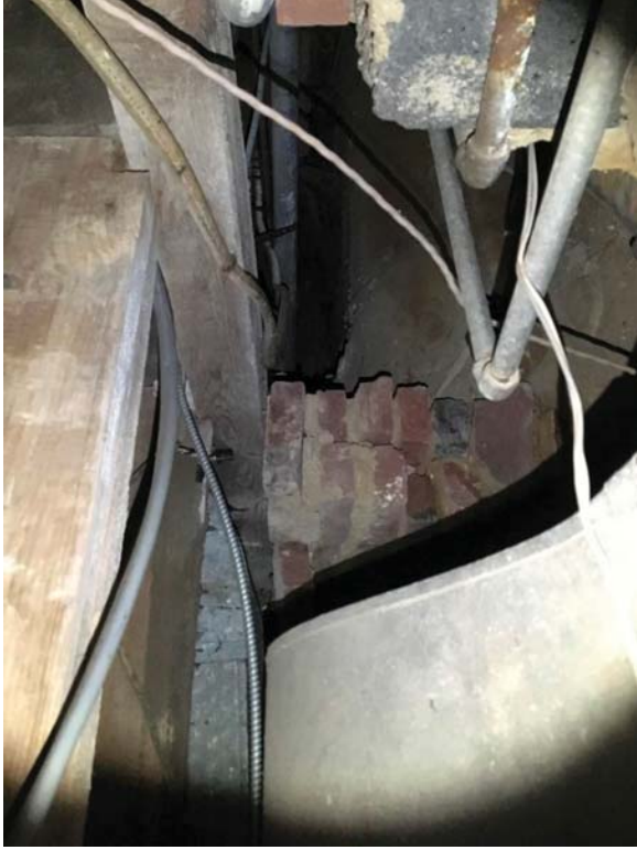
Crawl space under main portion of structure. Significant deterioration of masonry support.
