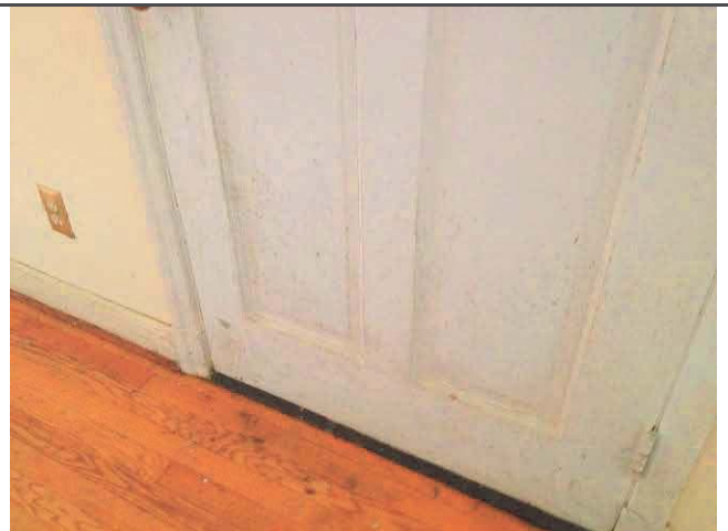
12. View of visible mold on the doors in the living room area.
