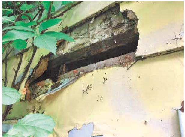
Door Frame damaged
