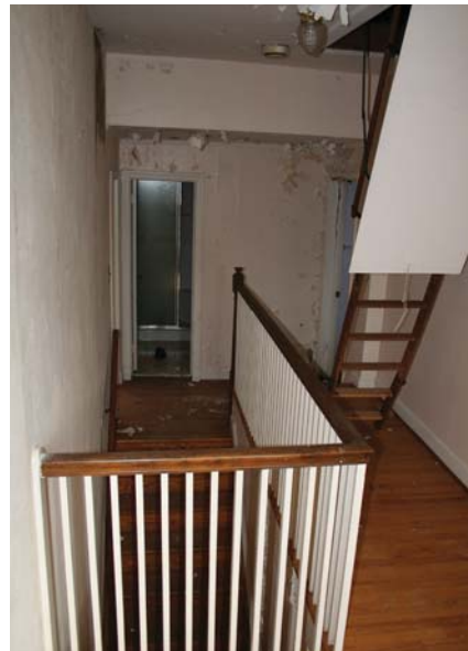
View of damaged finishes and attic access in Second Floor hallway
