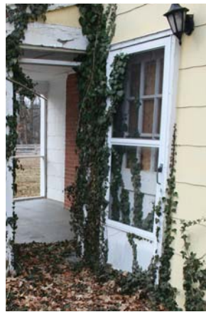
View of screen door of exterior door from Patio 1 into Family Room
