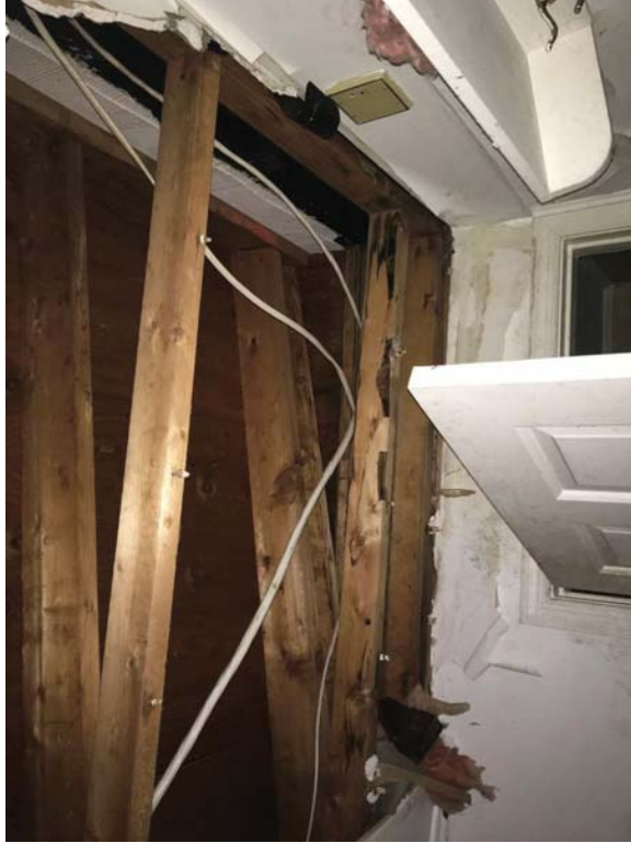
Collapsed ceiling observed on First Floor caused by water infiltration.
