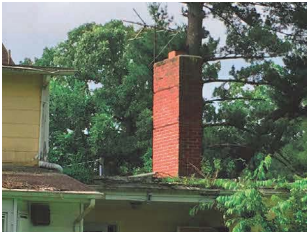
Gutters filled with debris
