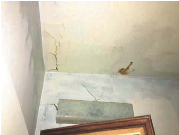
Cracks on a ceiling
