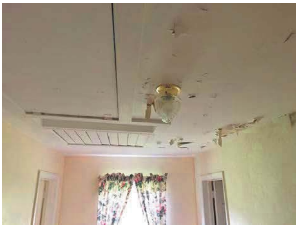
Second floor hallway ceiling sag
