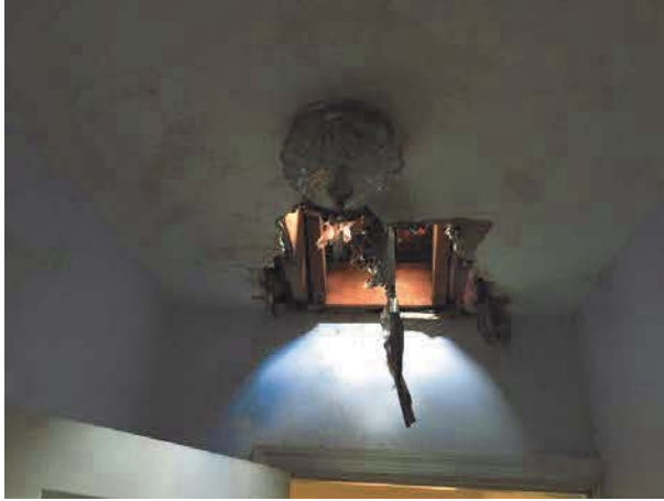
Hole in Roof
