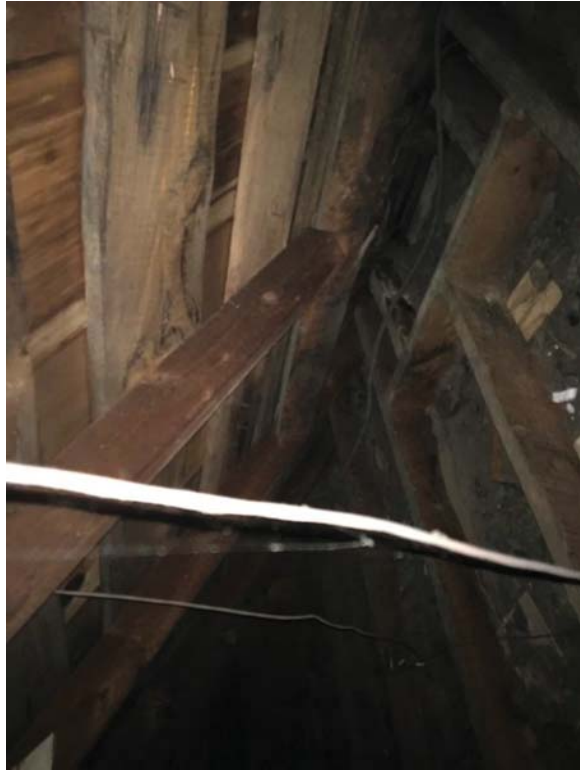
Water infiltration at roof framing. Partial failure of wood framing.
