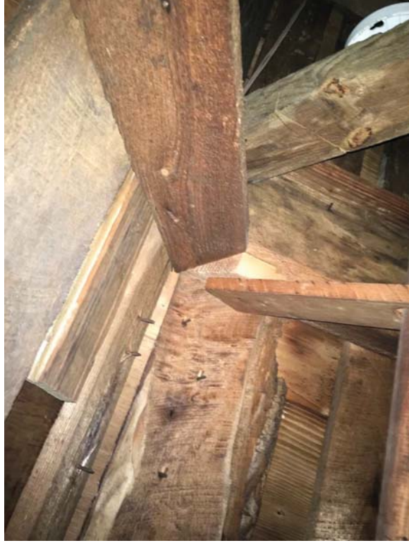
Roof rafters have displaced out of plane along ridge.
