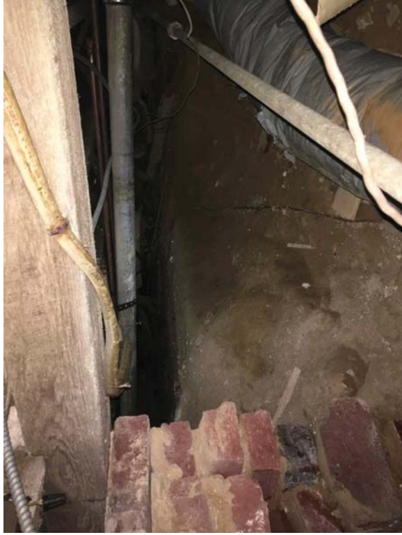
Significant deterioration of masonry foundation.
