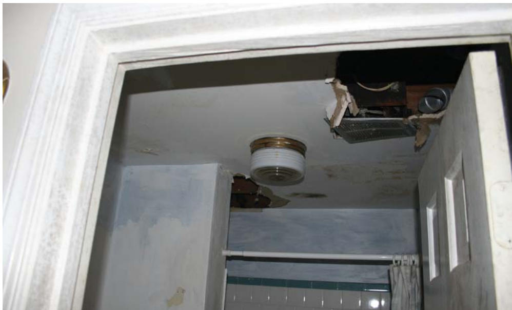
View of ceiling damage in 1st floor bathroom
