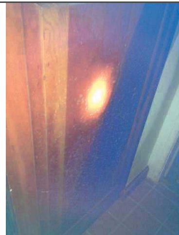
6. View of visible mold on kitchen cabinets.
