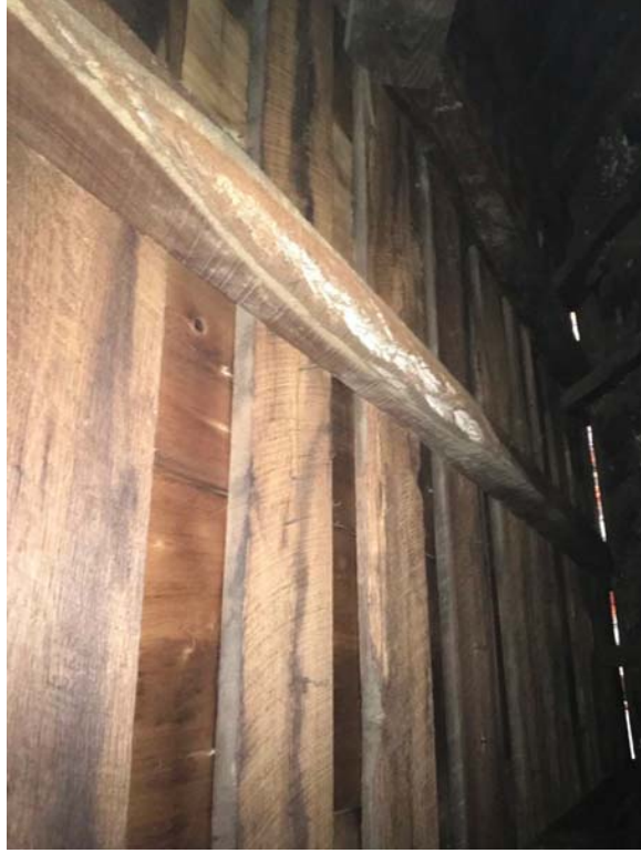
Wood framing appear bowed and twisted.
