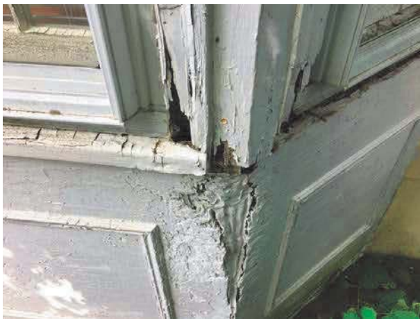
Window frame wood rot
