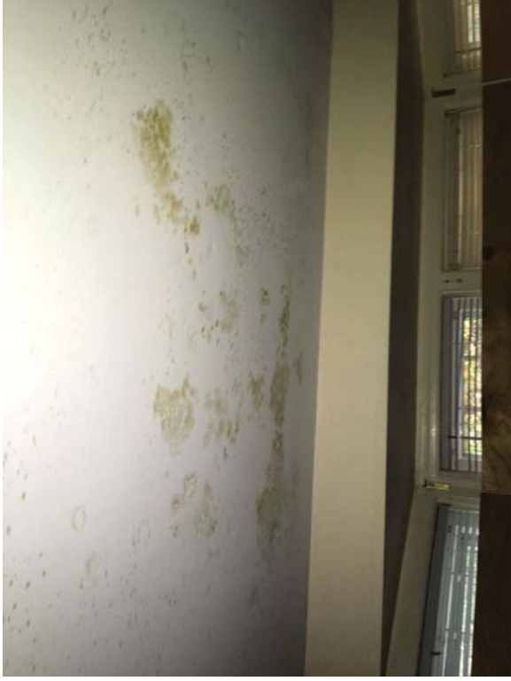
Peeling paint and mold growth.
