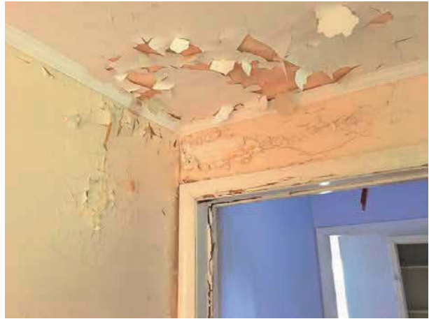
Ceiling paint peeling
