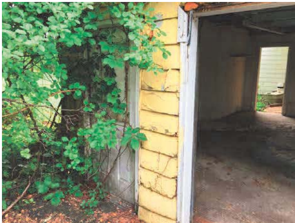
Door Frame damaged
