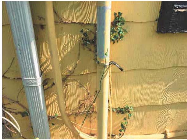
Organic on the wall
