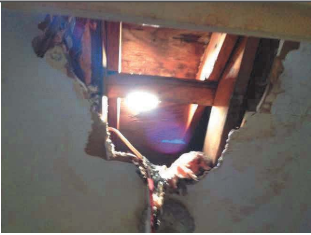
7. View of the hole in the roof at the 2 nd floor stairwell hallway.
