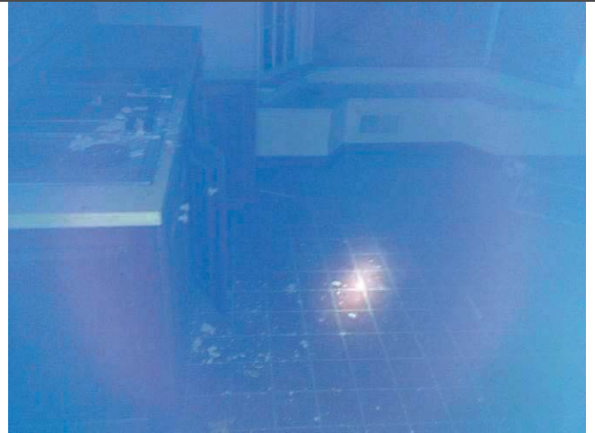
16. View of ceiling debris (with asbestos) on the floor in the kitchen.
