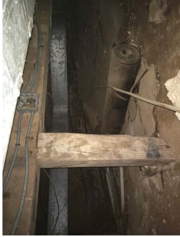
Wood post with crawl space, supporting floor. Wood deterioration.
