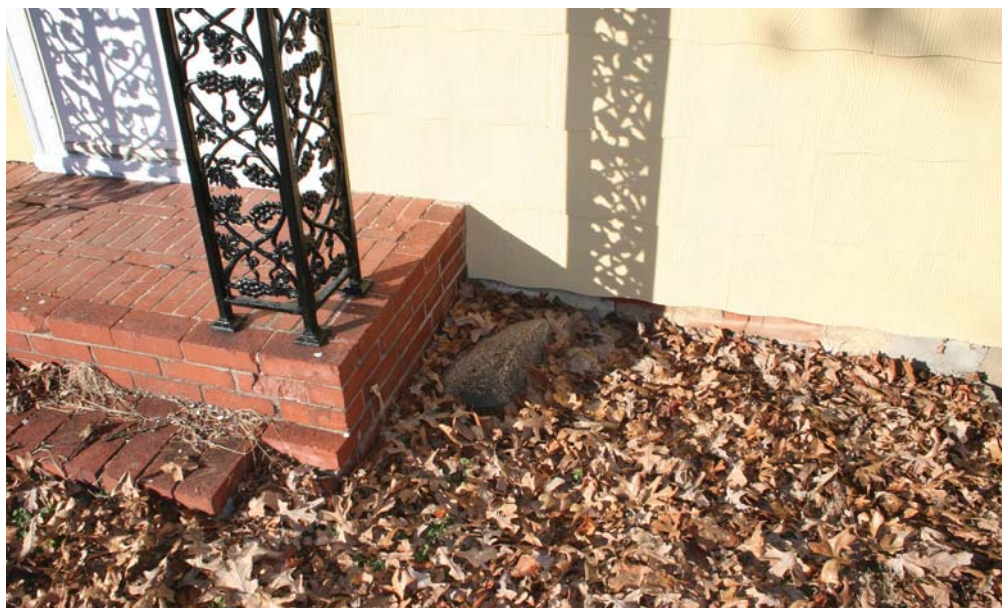
View of front brick steps, note missing corner
