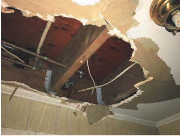
Hole in Laundry Room
