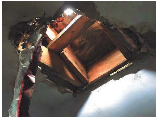
Hole in Roof
