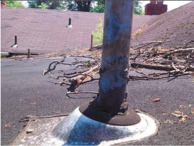
21. View of the cement (ACM) on the roof vent, Samples 67-68
