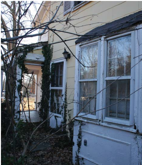
View of overgrown East
