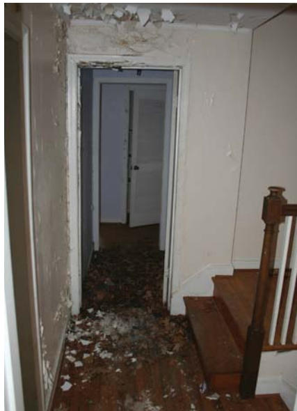
View of damaged finishes in Second Floor Hallway
