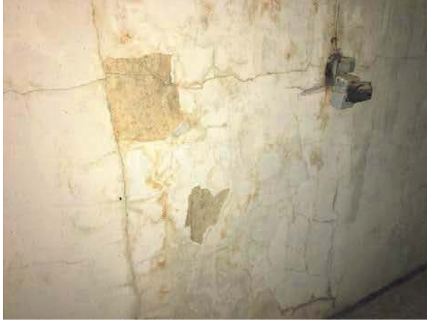
Cracks in the parged walls
