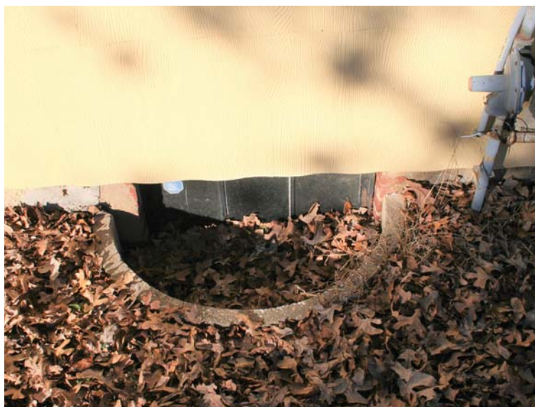
View of window well into the basement and yellow shingles on the South facade
