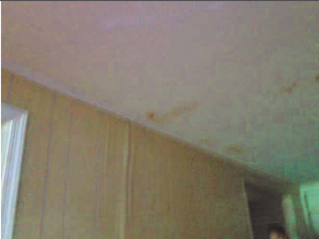
15. View of water impacted walls and ceiling in the northeast living room.
