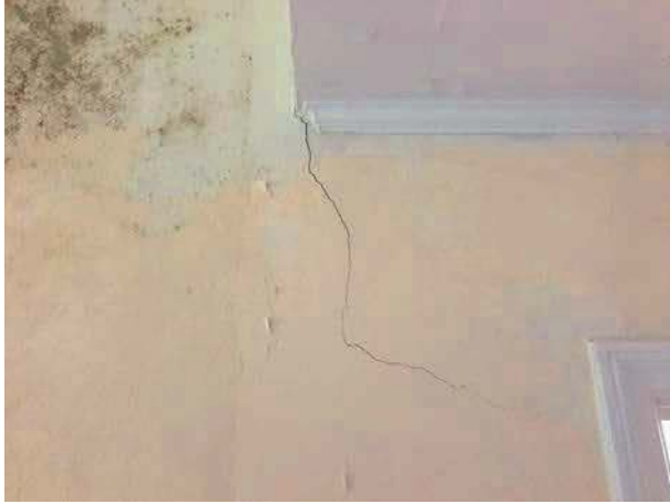
Crack along a wall
