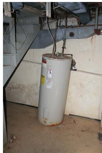
View of basement water heater
