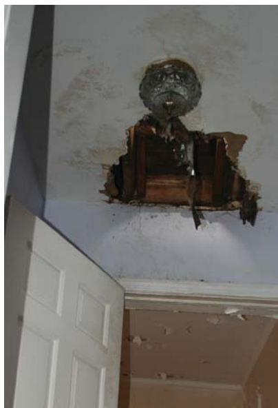
View of hole in roof on 2nd floor
