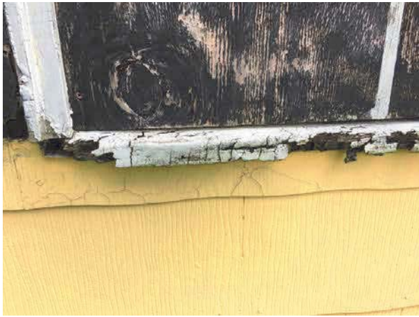
Window frame wood rot
