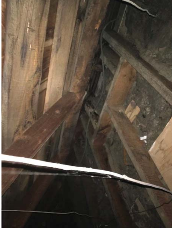
Partial failure of roof framing.
