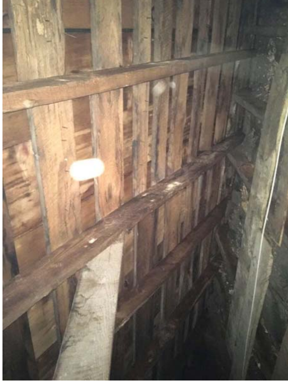
Base of roof rafters appear to have displaced outward. Wood framing appear bowed and twisted.
