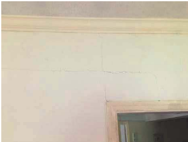
Cracks along a wall
