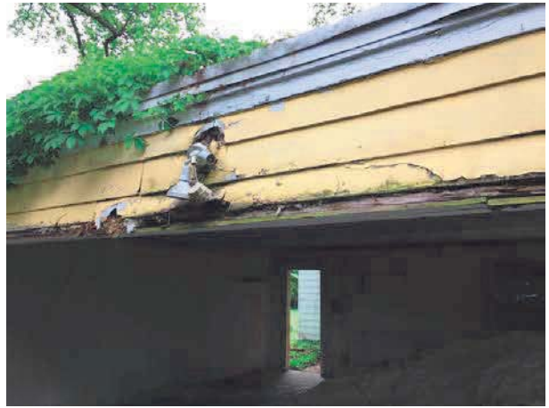
Door Frame damaged
