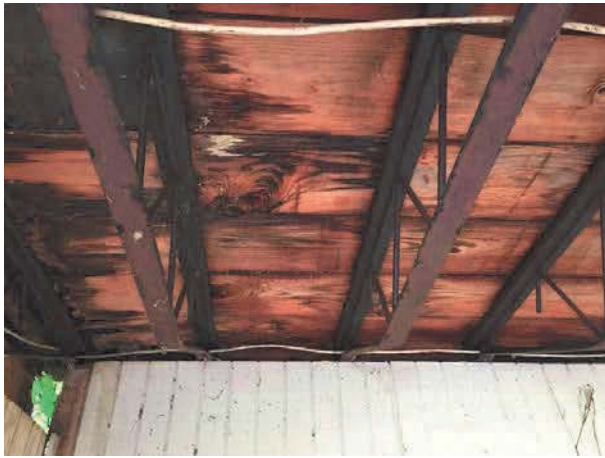
Wood roof water damaged
