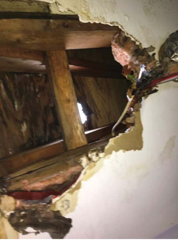
Partial collapse of roof structure.
