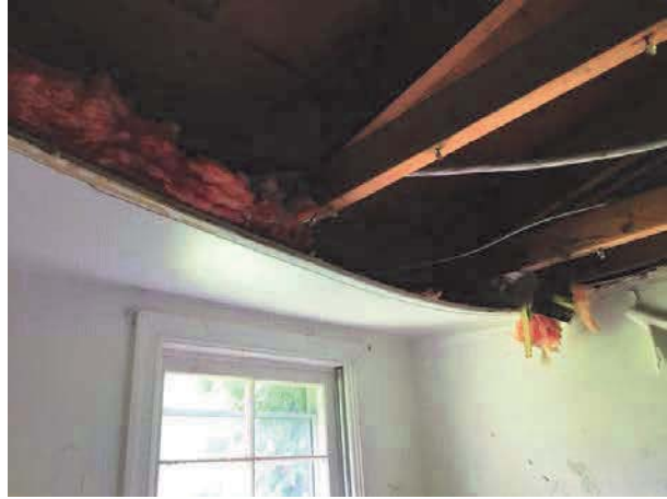
Hole in Laundry Room
