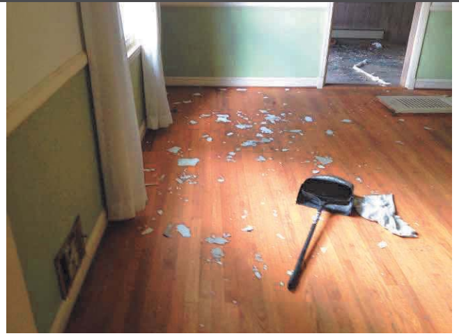
14. View of peeling paint on the floor surfaces.
