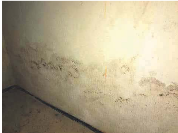
Water damage of the walls
