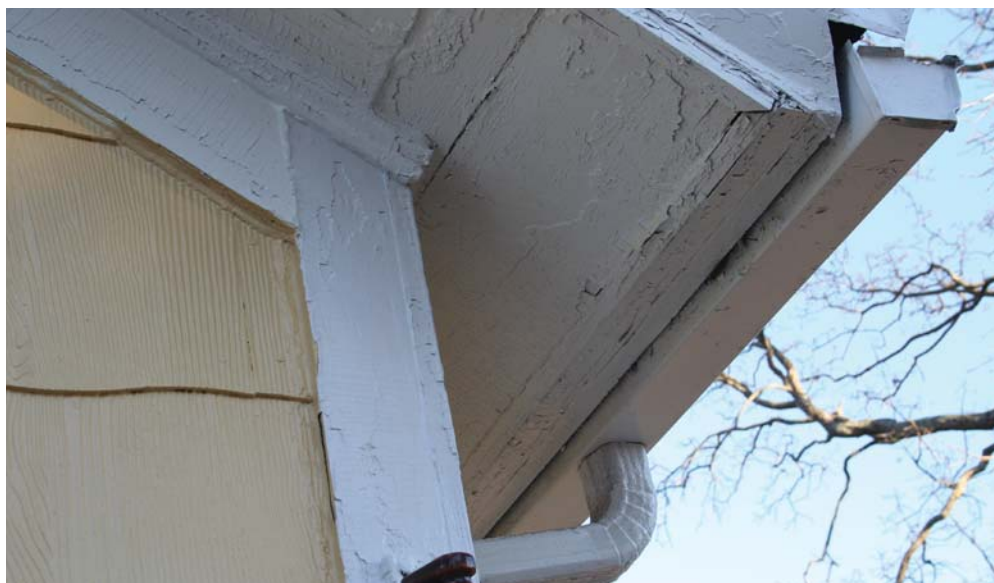
View of fascia, gutter, and downspout at the Southwest corner of the original structure
