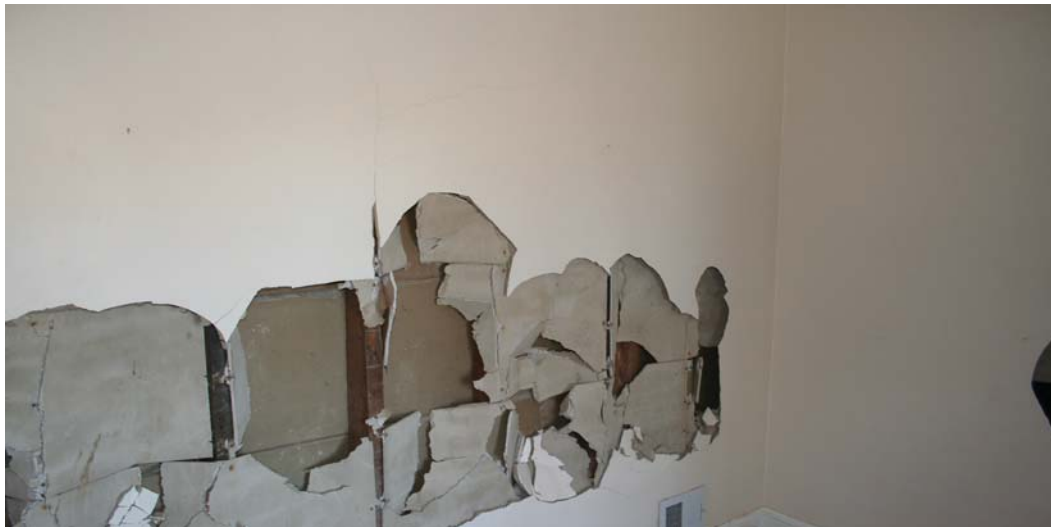
View of damaged drywall in Bedroom 3
