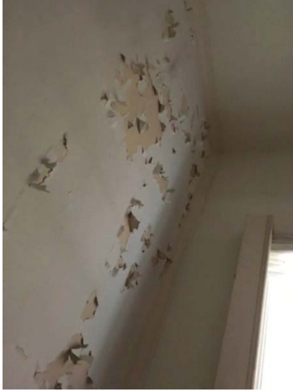
Peeling paint typical throughout building.
