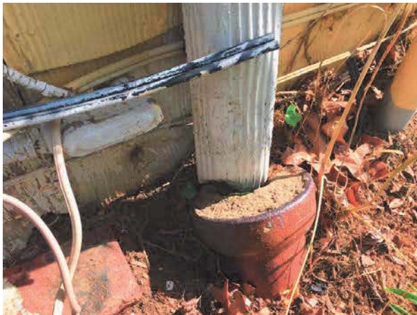
Downspout path blocked
