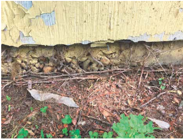
Organic grow into the wall
