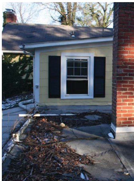
View of debris on garage roof
