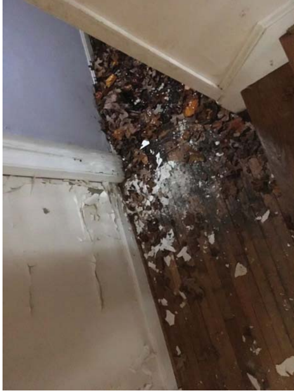
Floor debris at partial collapse of roof structure.
