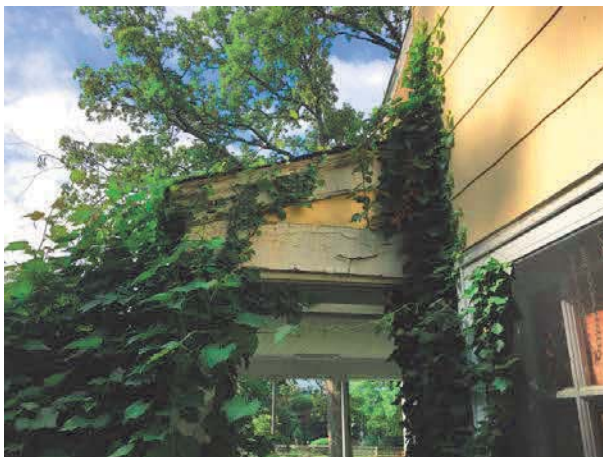
Growth on side porch
