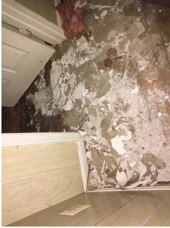
Collapsed ceiling debris on floor.
