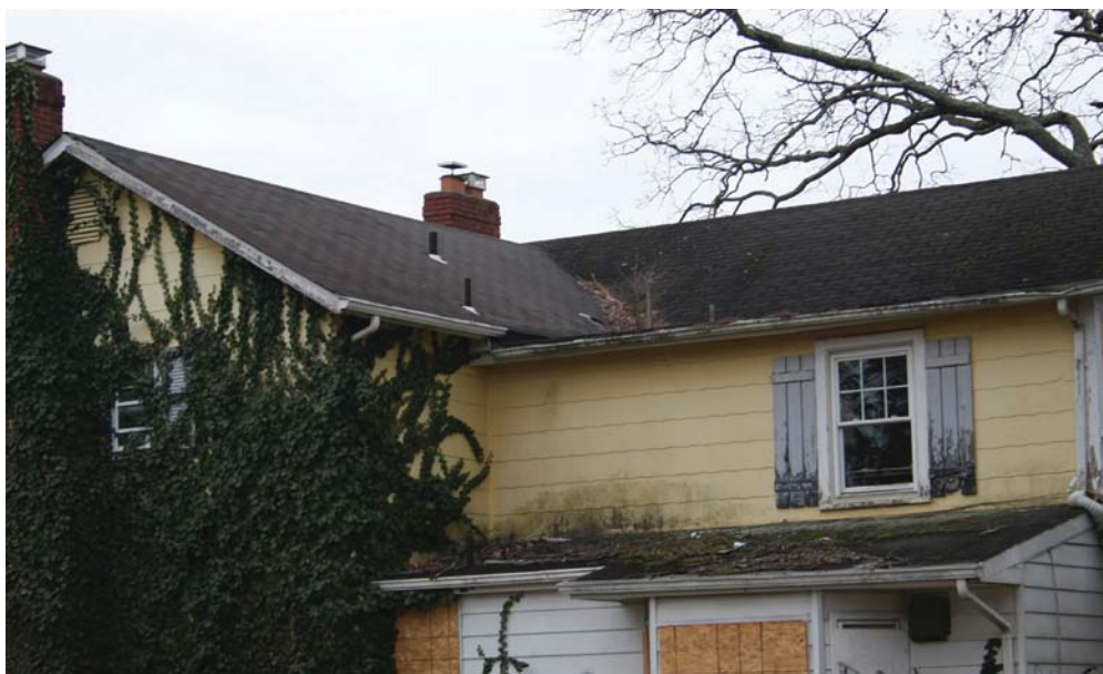
View of organic growth on building and in gutters
