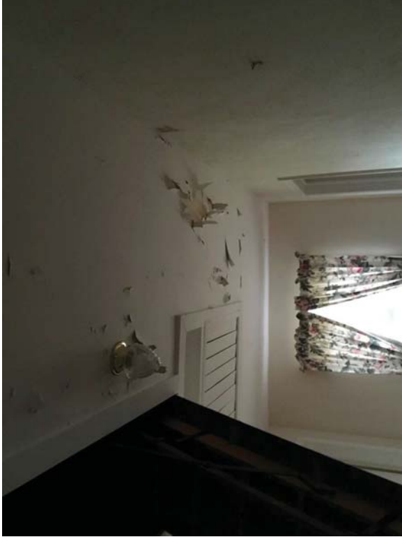
Peeling paint typical throughout building.
