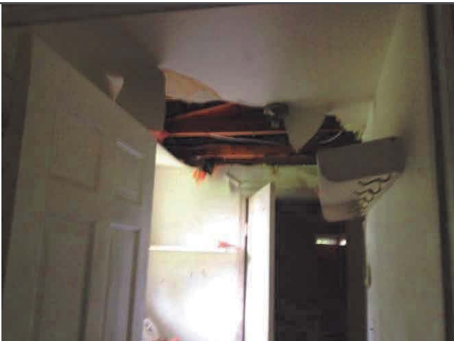
17. View of the ceiling damage from a roof leak in the laundry room/hall.
