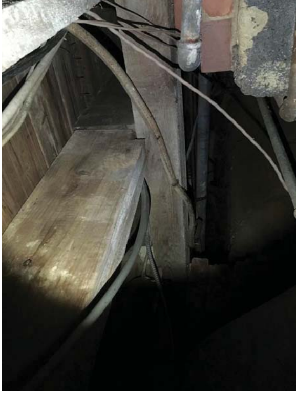
Displacement of floor beam. Beam appears undersized.
