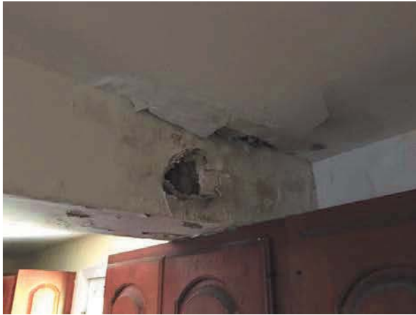
Water damaged drywall in kitchen
