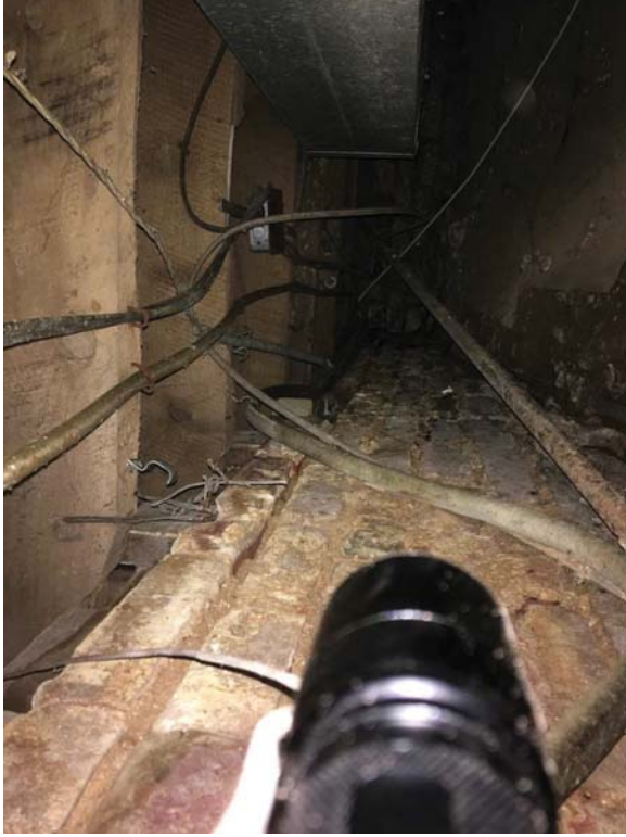
Significant deterioration of masonry foundation.
