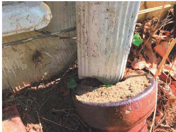
Downspout path blocked
