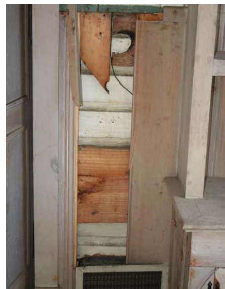
View of covered exterior German siding from 1911 portion of house behind Den door into Dining Room
