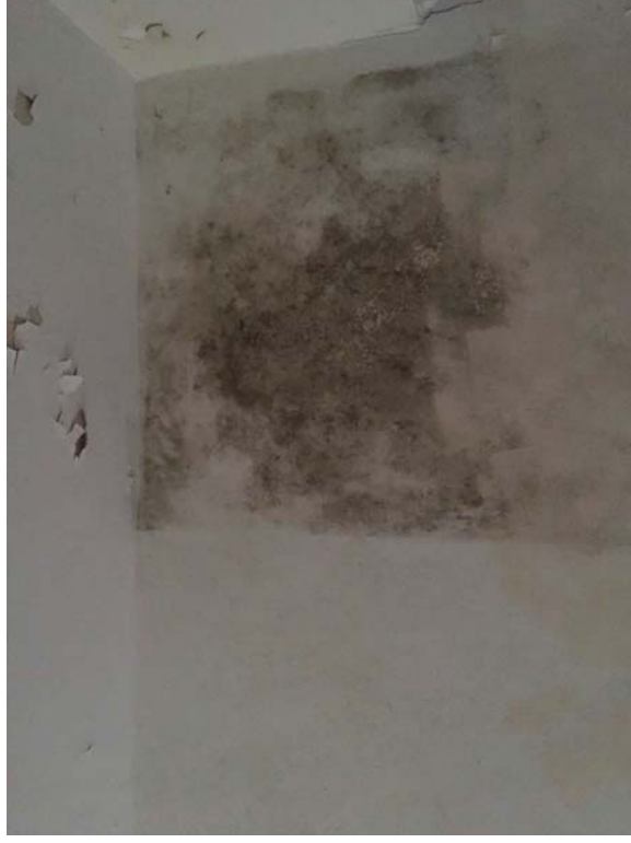
Peeling paint and mold growth.
