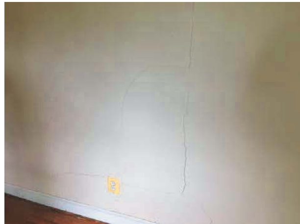
Cracks along a wall
