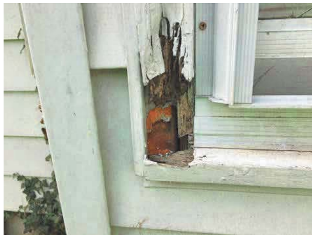
Window frame wood rot
