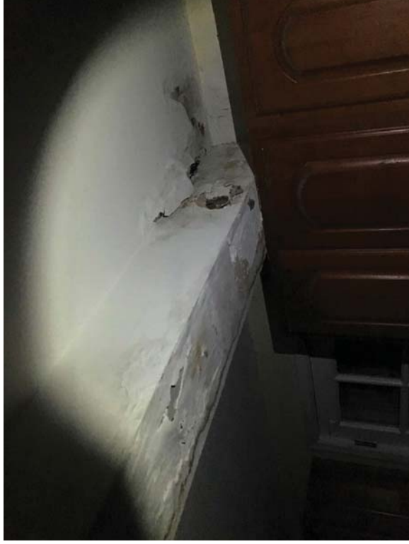
Water damage to finishes.
