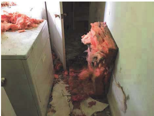
Insulation from ceiling in laundry room exposed
