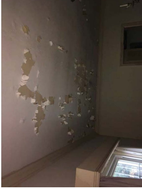
Peeling paint typical throughout building.
