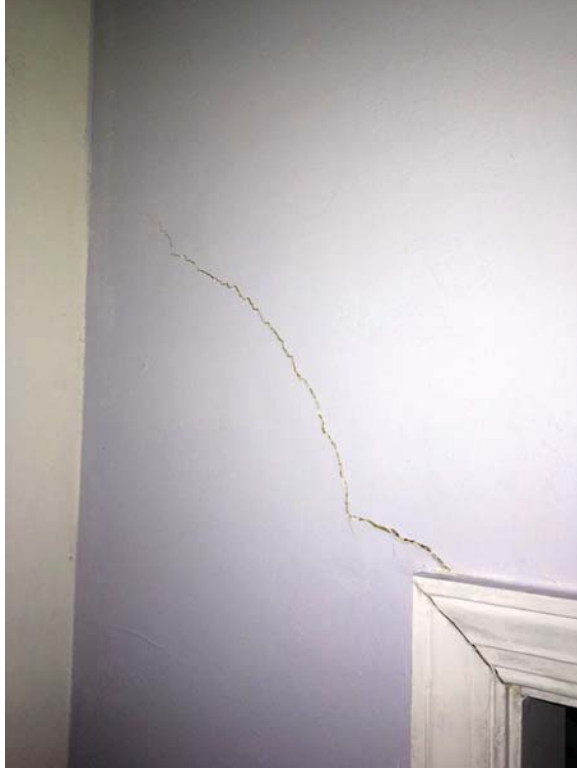
Typical diagonal cracking through wall finish at opening corners.
