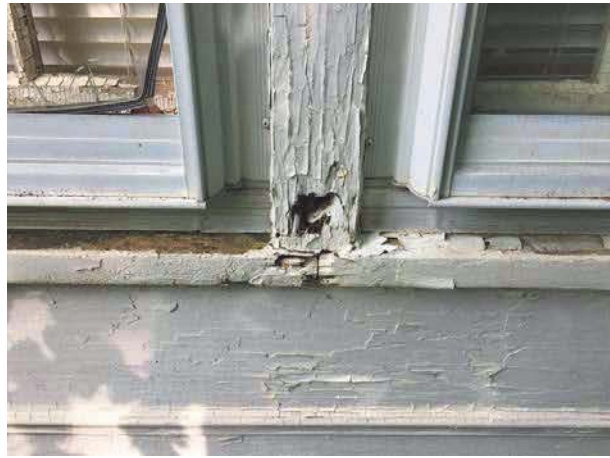
Window frame wood rot
