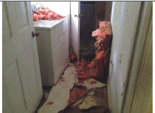
18. View of impacted materials from a roof leak in the laundry room/hall.
