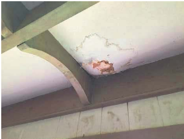
Water damage on ceiling in room adjacent to garage
