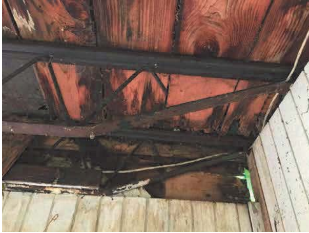
Steel surface rusted
