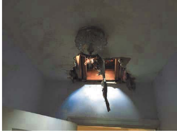
Hole penetrating from roof
