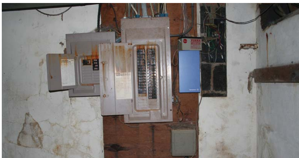
View of Electrical panels in basement
