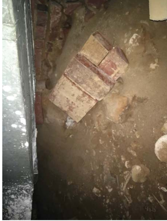
Partial collapse of masonry foundation.
