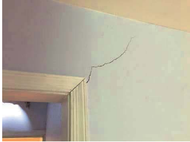
Crack along a wall
