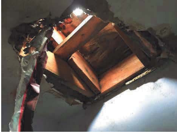
Hole penetrating from roof
