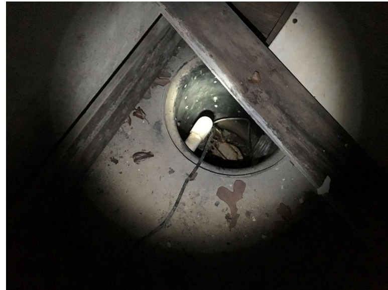
Sump pit within Cellar level. Pit was dry.
