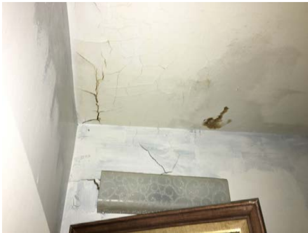
Cracks on a ceiling
