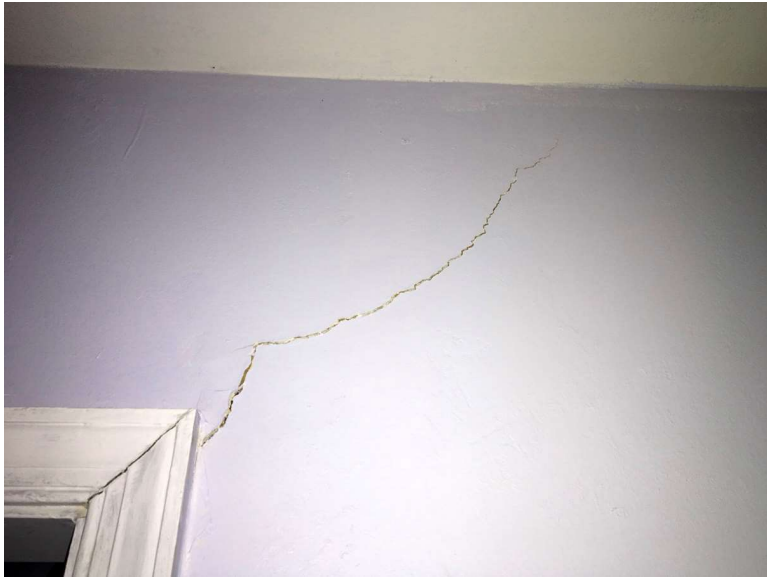
Typical diagonal cracking through wall finish at opening corners.
