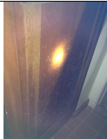
6. View of visible mold on kitchen cabinets.
