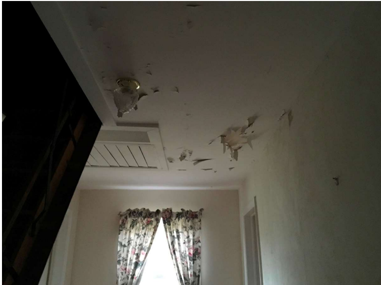
Peeling paint typical throughout building.
