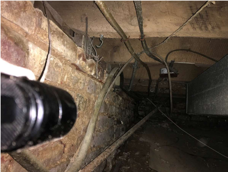
Significant deterioration of masonry foundation.
