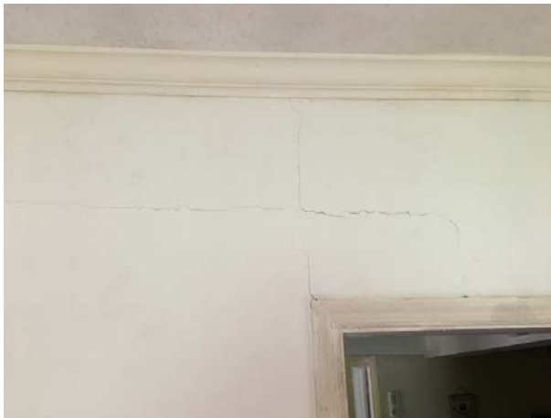
Cracks along a wall
