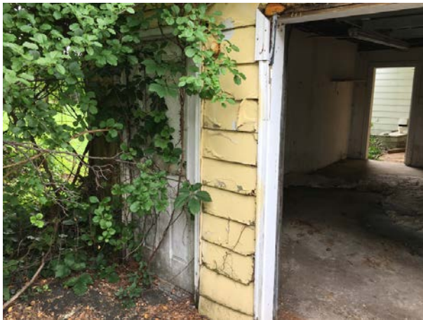
Door Frame damaged
