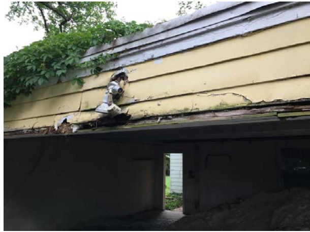
Door Frame damaged
