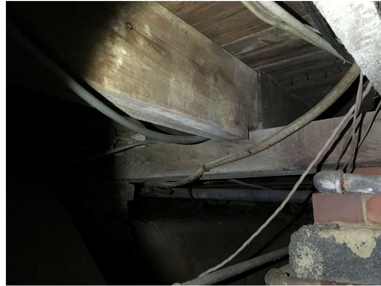
Displacement of floor beam. Beam appears undersized.
