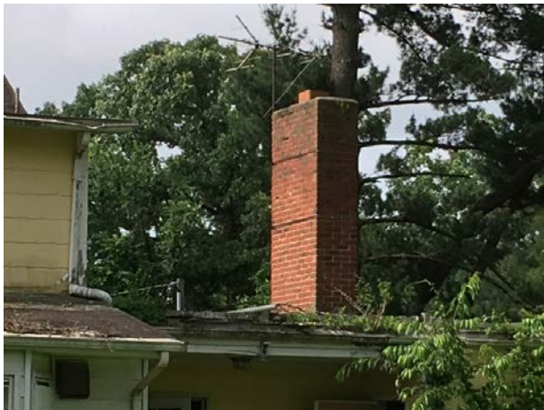
Gutters filled with debris
