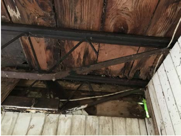
Steel surface rusted
