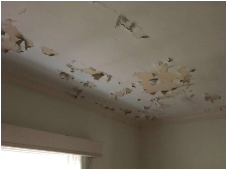
Peeling paint typical throughout building.
