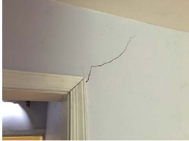
Crack along a wall
