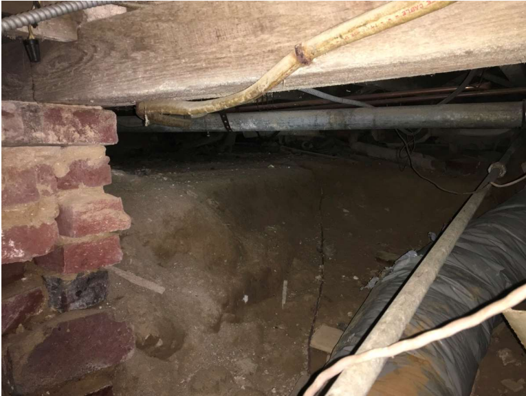
Significant deterioration of masonry foundation.
