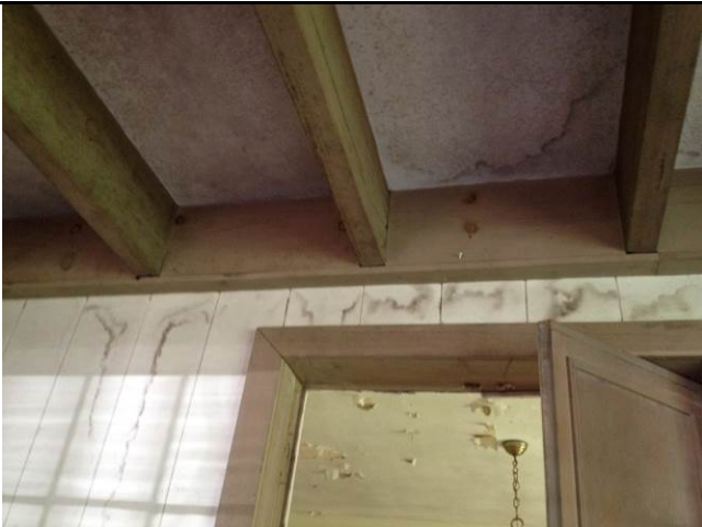
9. View of visible mold on the ceiling/walls in the den.
