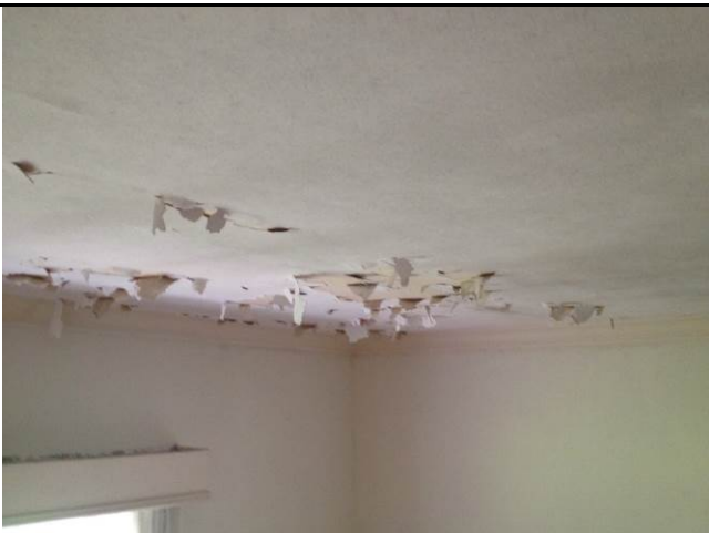
11. View of peeling paint in the dining room with mold on the ceiling.
