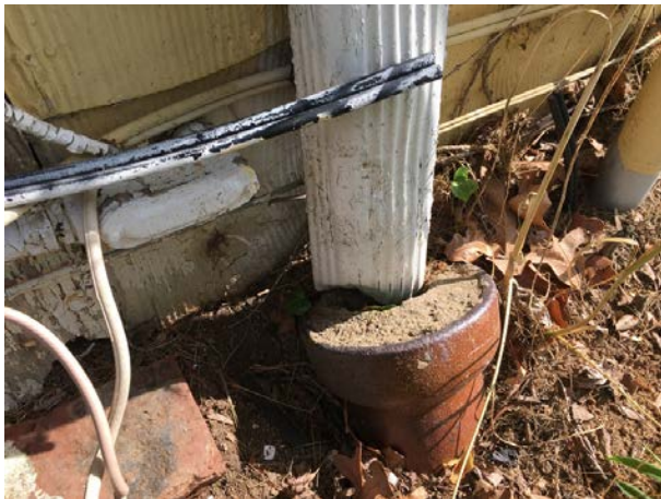
Downspout path blocked
