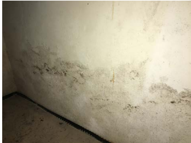
Water damage of the walls
