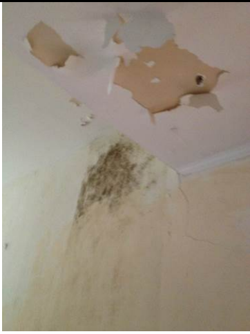
19. View of visible mold and peeling paint in the upstairs hallway.
