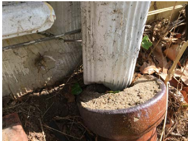
Downspout path blocked
