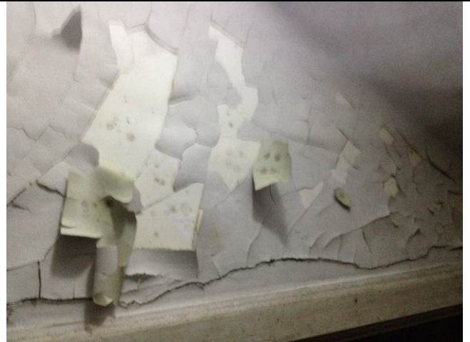
4. View of peeling paint with mold in the basement stairwell.
