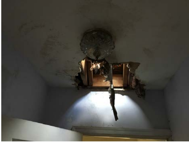
Hole in Roof
