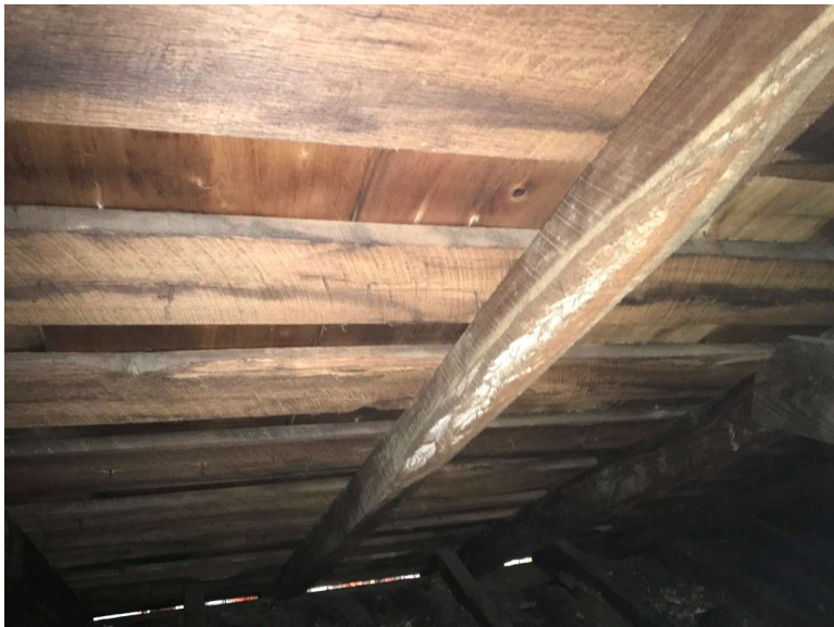
Wood framing appear bowed and twisted.
