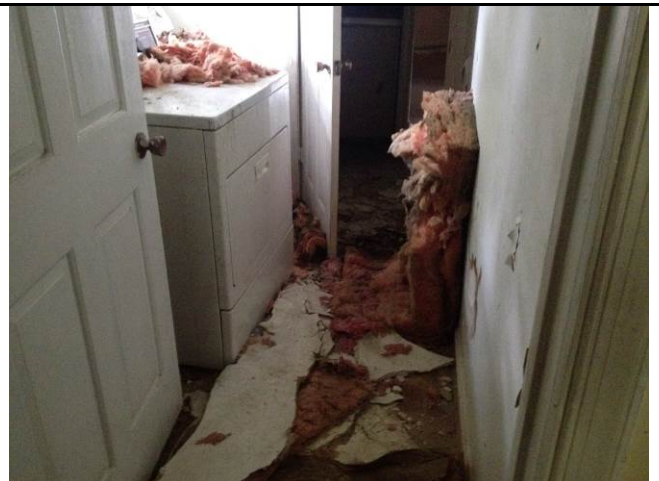
18. View of impacted materials from a roof leak in the laundry room/hall.
