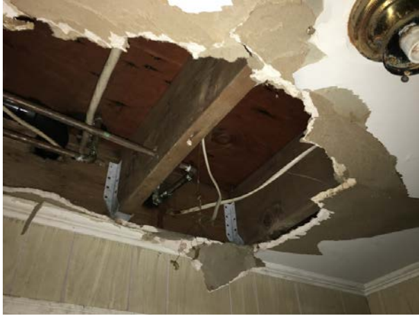
Hole in Laundry Room
