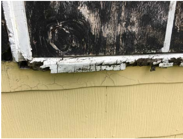
Window frame wood rot
