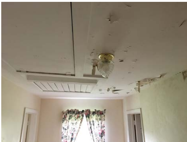
Second floor hallway ceiling sag
