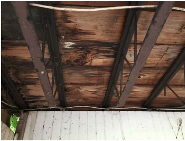
Wood roof water damaged
