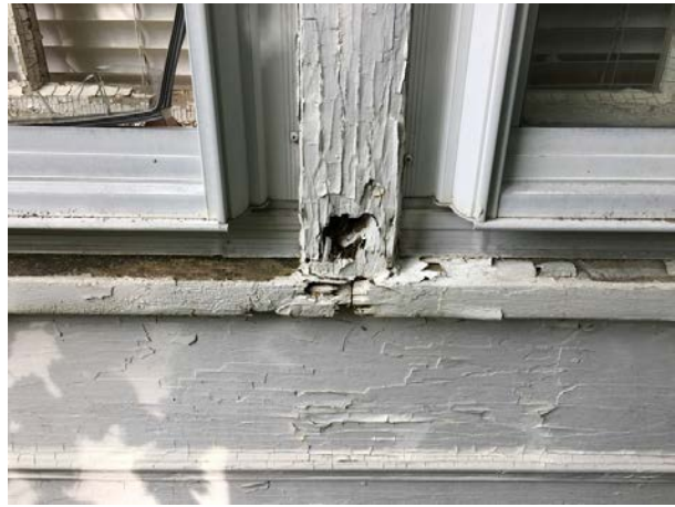
Window frame wood rot
