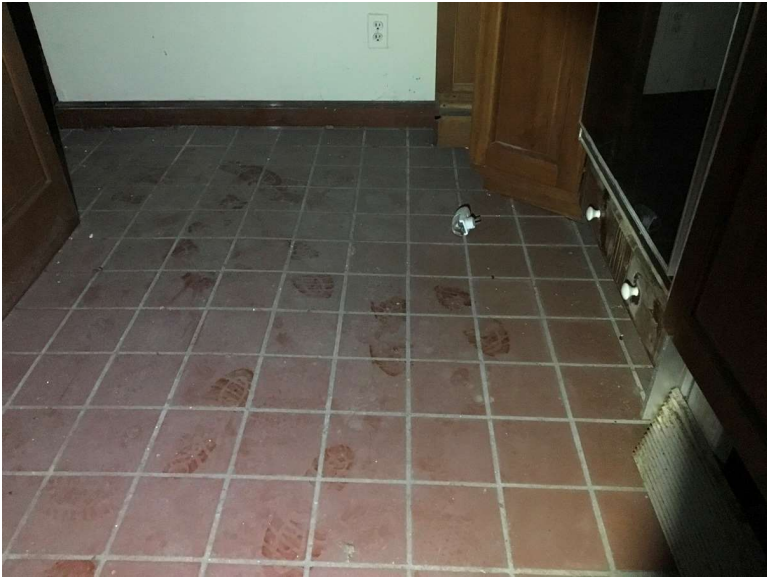
Significant displacement of floor structure within kitchen. Estimated 1.5" within five feet.
