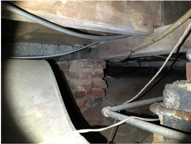
Crawl space under main portion of structure. Significant deterioration of masonry support.
