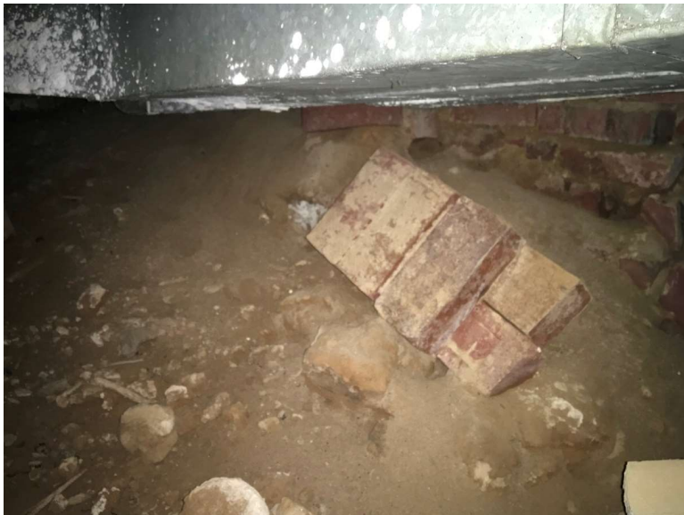
Partial collapse of masonry foundation.
