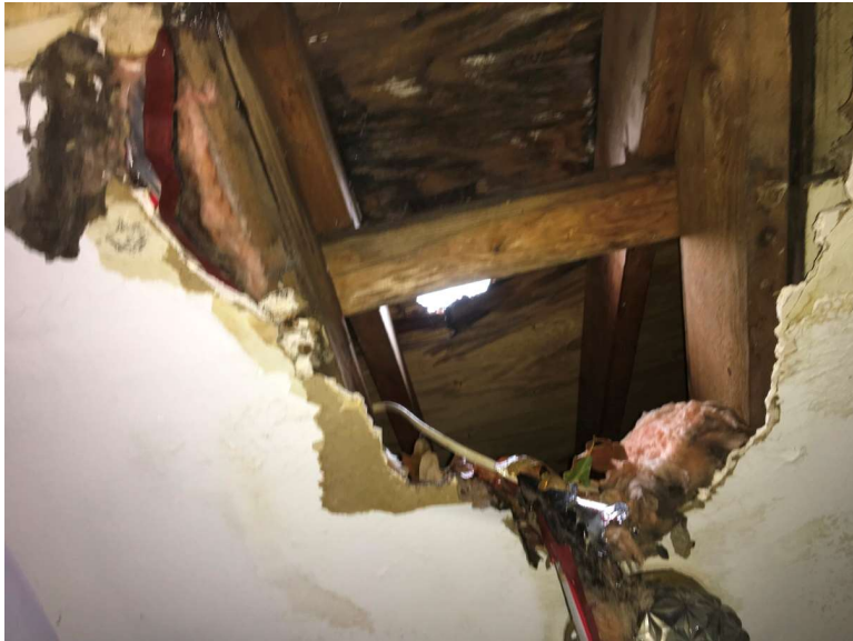
Partial collapse of roof structure.
