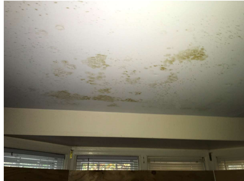
Peeling paint and mold growth.
