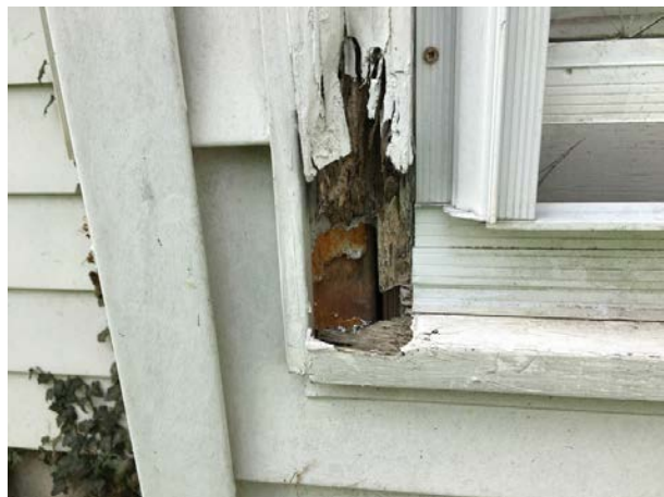
Window frame wood rot
