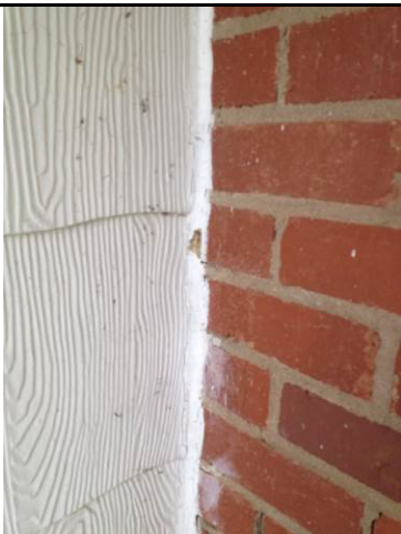
23. View of the tan caulk (ACM) on the chimney of the patio.
