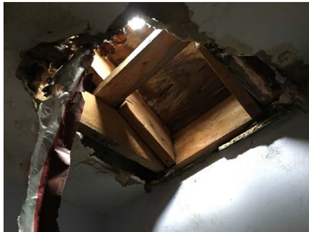
Hole in Roof
