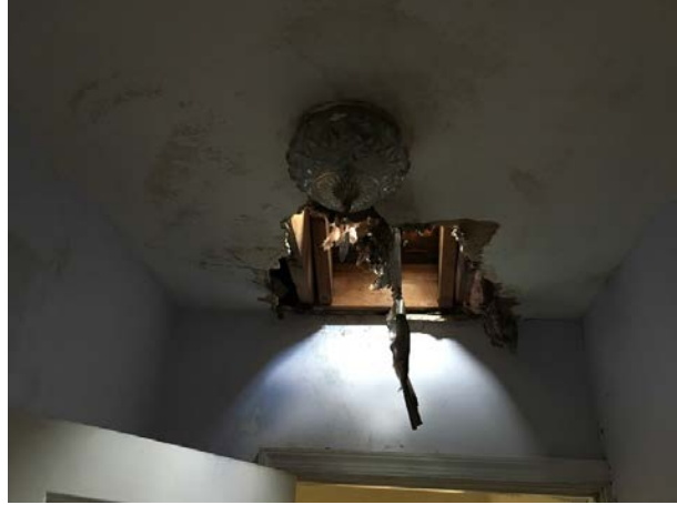
Hole penetrating from roof
