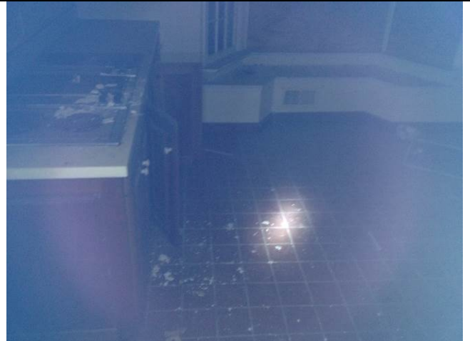
16. View of ceiling debris (with asbestos) on the floor in the kitchen.
