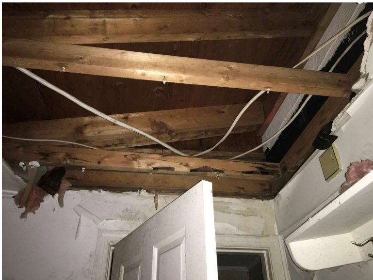
Collapsed ceiling observed on First Floor caused by water infiltration.
