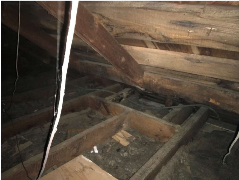
Partial failure of roof framing.
