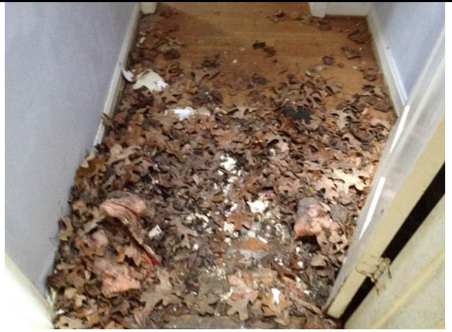
8. View of debris on the floor, partial hole in the floor from the roof leak.
