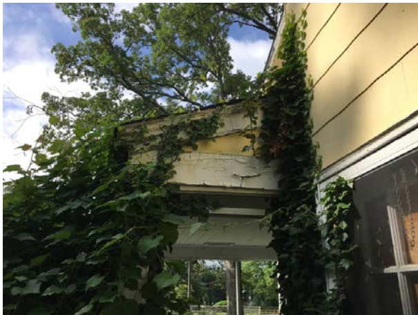
Growth on side porch
