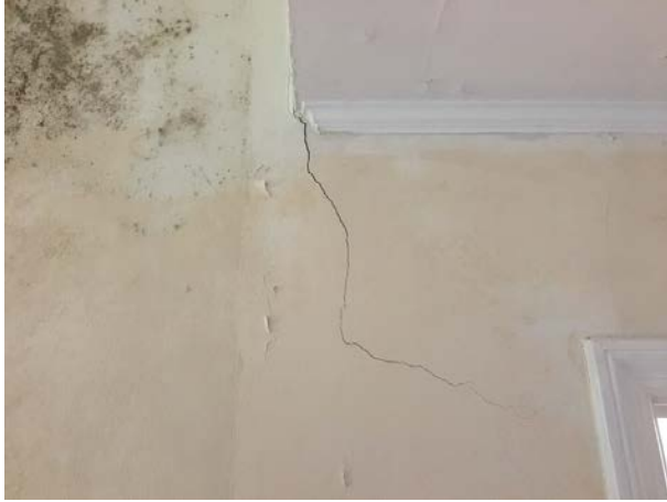
Crack along a wall
