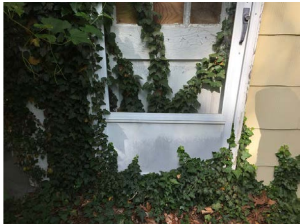
Growth on side door near porch
