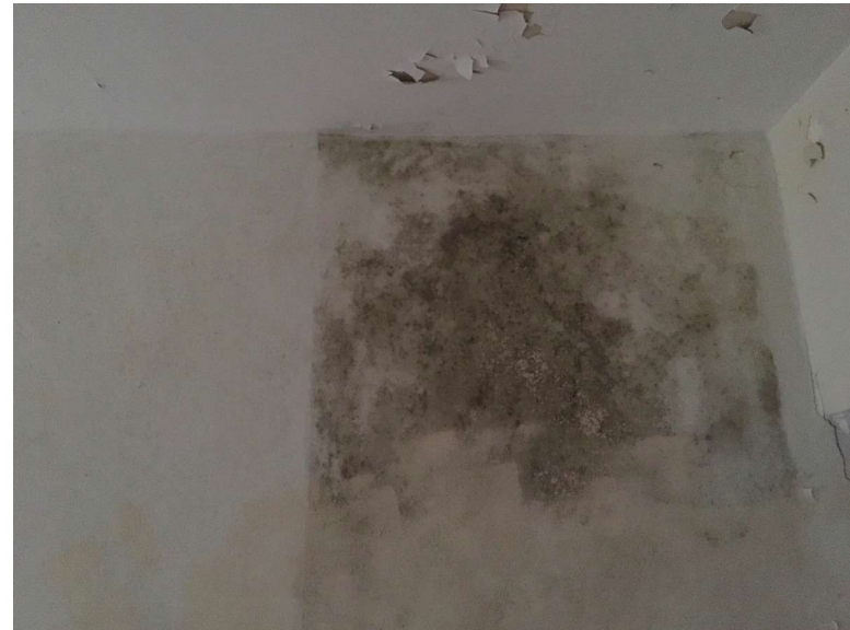
Peeling paint and mold growth.
