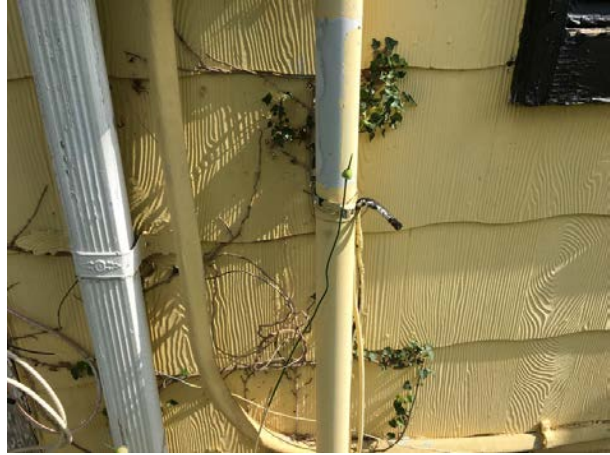
Organic on the wall
