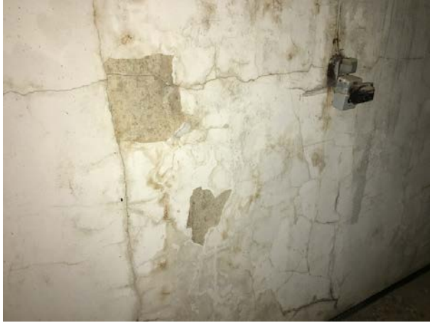
Cracks in the parged walls
