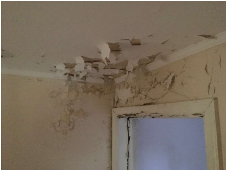
Peeling paint typical throughout building.
