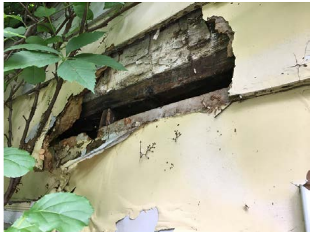
Door Frame damaged
