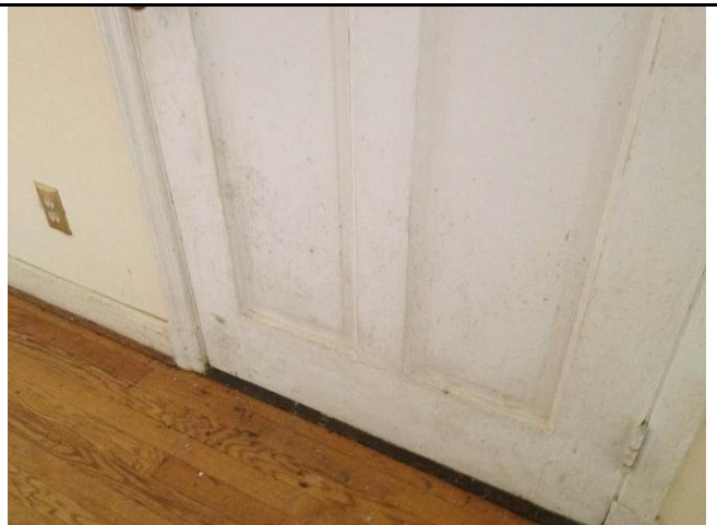
12. View of visible mold on the doors in the living room area.
