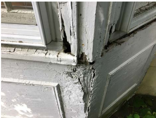
Window frame wood rot
