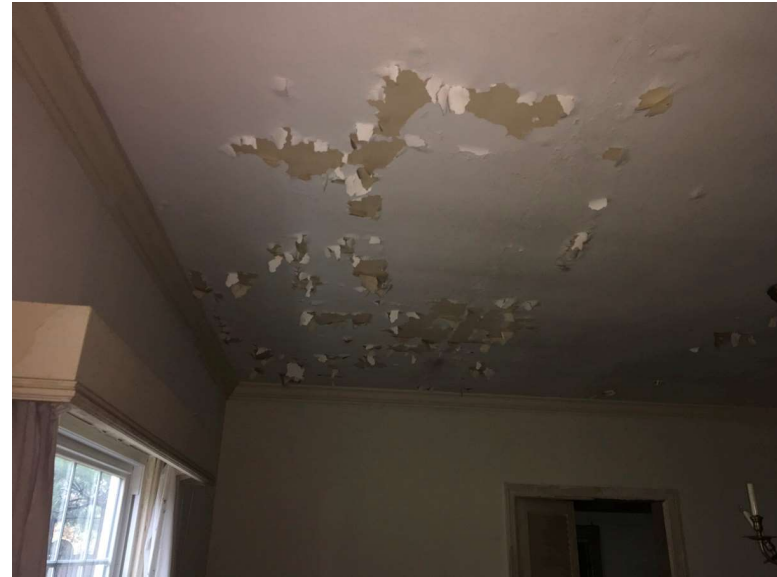
Peeling paint typical throughout building.
