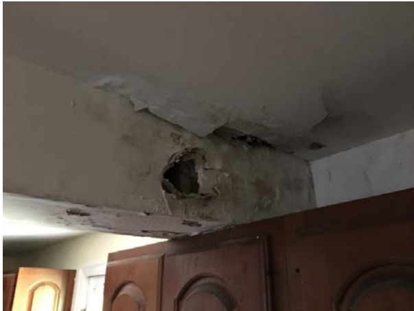
Water damaged drywall in kitchen
