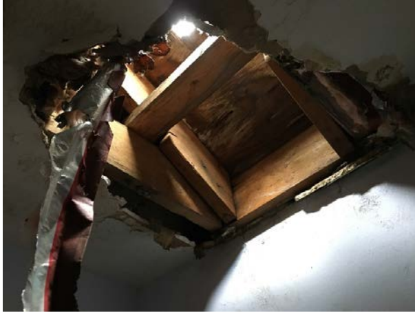
Hole penetrating from roof
