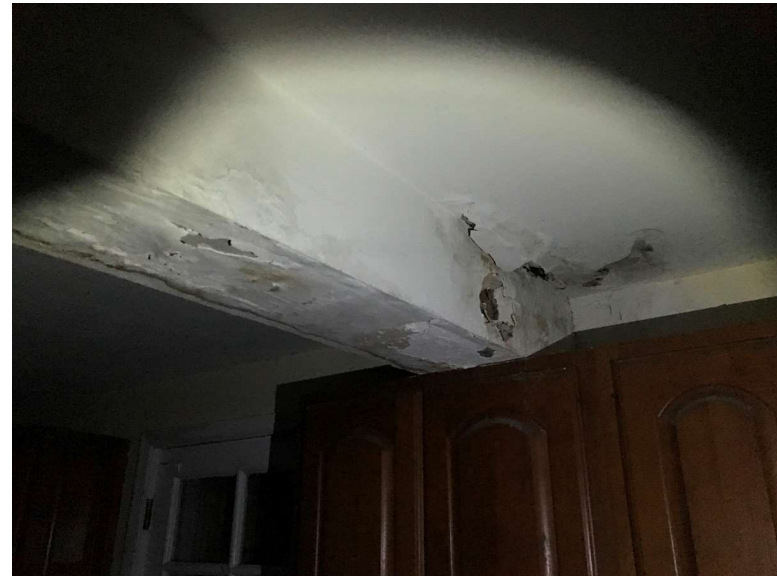
Water damage to finishes.
