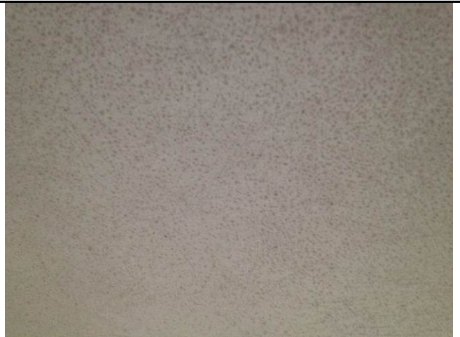
10. View of visible mold on the ceiling in the dining room.
