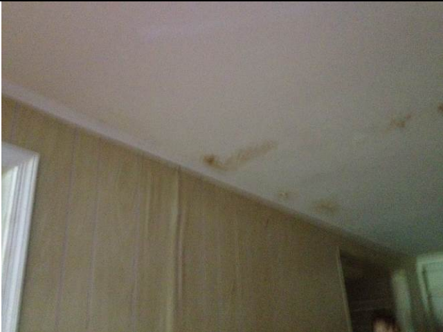
15. View of water impacted walls and ceiling in the northeast living room.
