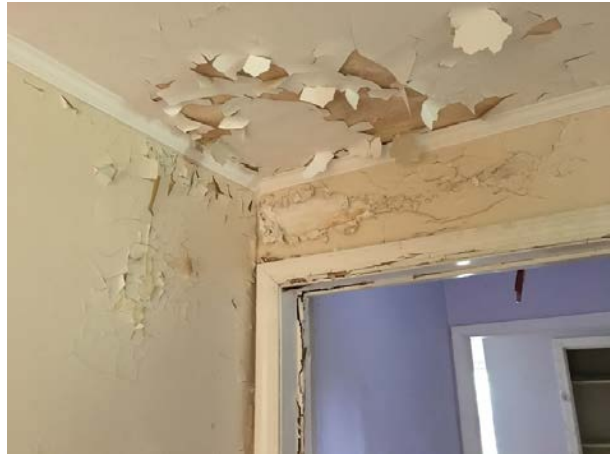
Ceiling paint peeling
