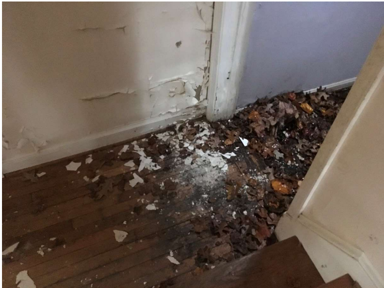
Floor debris at partial collapse of roof structure.
