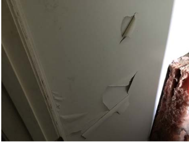
Paint peeling from wall in laundry room
