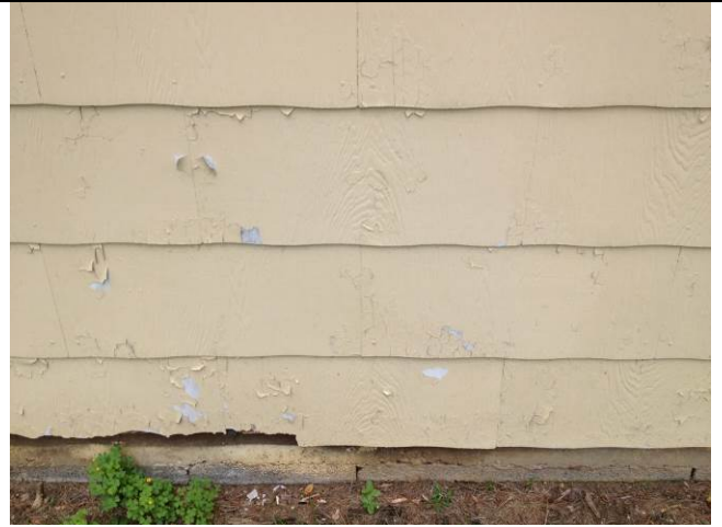
22. View of the cement board siding (ACM), Samples 73-74, and paint chips in the drip line.
