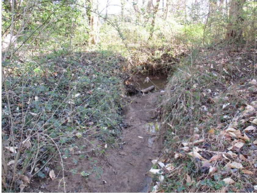
Figure 5. Eroded pond inflow channel (2016)
