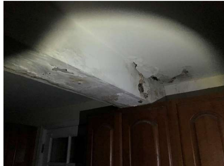
Water damage to finishes.
