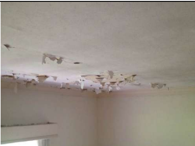
11. View of peeling paint in the dining room with mold on the ceiling.
