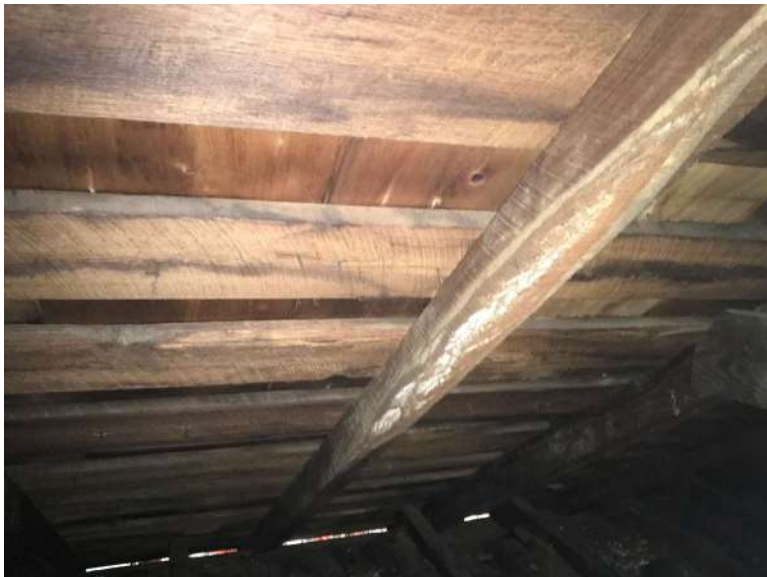
Wood framing appear bowed and twisted.
