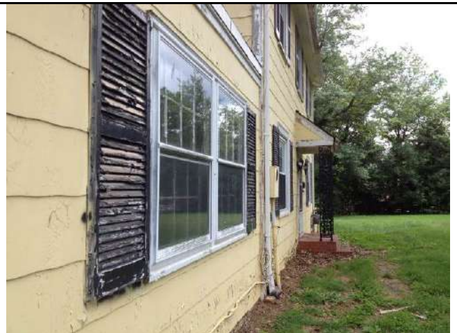
24. View of peeling paint (LBP) on the exterior of the house.
