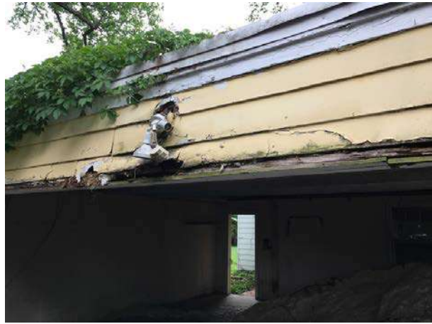
Door Frame damaged
