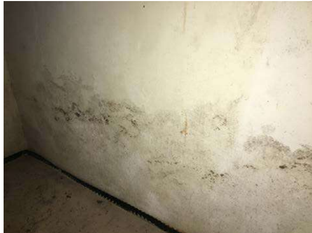
Water damage of the walls
