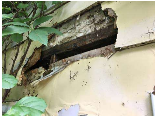
Door Frame damaged
