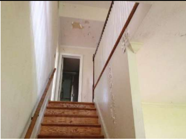
13. View of peeling paint on the walls and ceiling.
