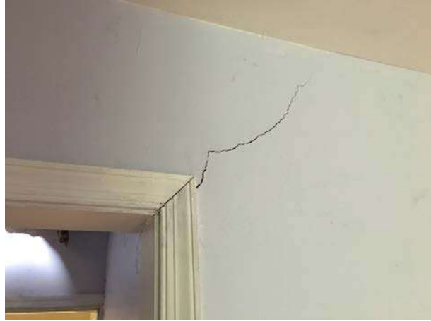
Crack along a wall
