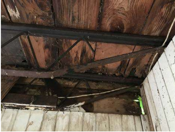
Steel surface rusted
