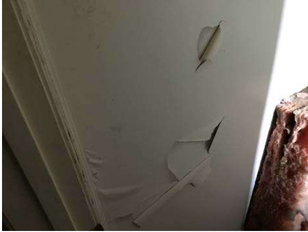
Paint peeling from wall in laundry room
