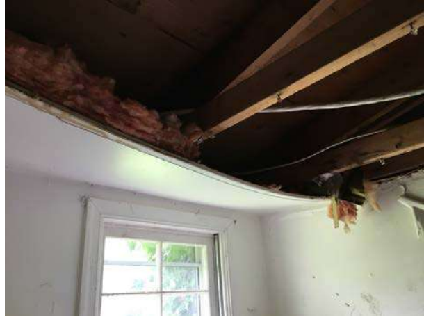
Hole in Laundry Room
