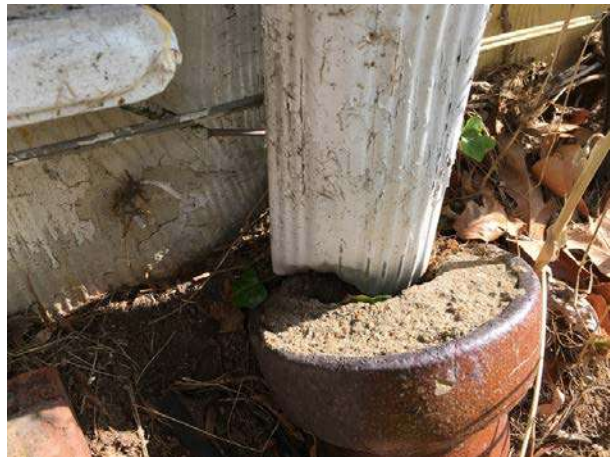
Downspout path blocked
