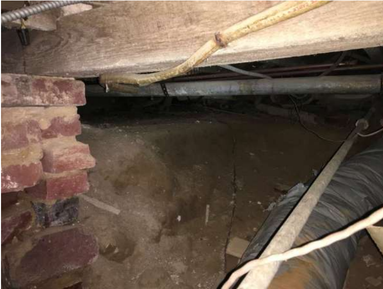
Significant deterioration of masonry foundation.
