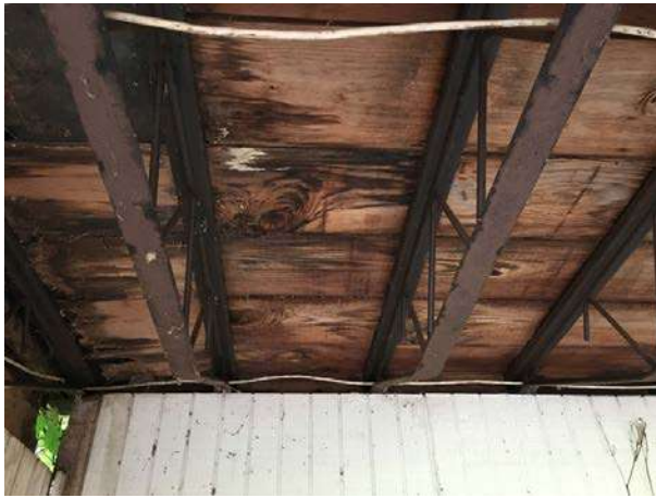
Wood roof water damaged
