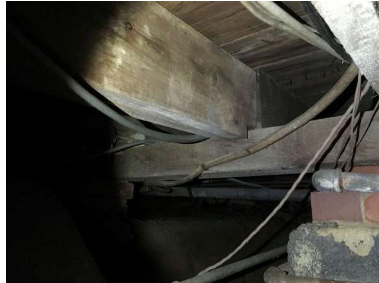
Displacement of floor beam. Beam appears undersized.
