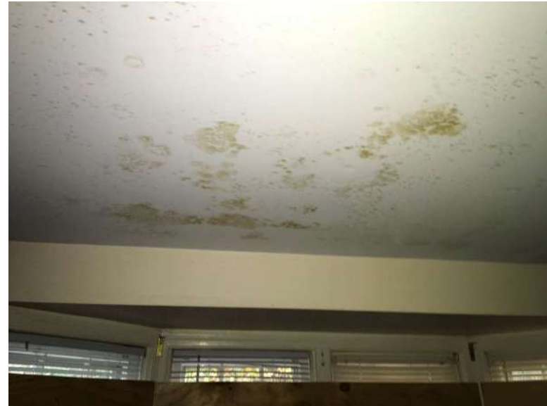
Peeling paint and mold growth.
