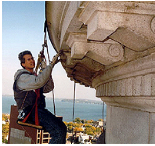
The use of special access methods may be necessary for close-up investigation of building elements. At the Wisconsin State Capitol, project architects and engineers used rappelling techniques. Photo: Wiss, Janney, Elstner Associates, Inc.
