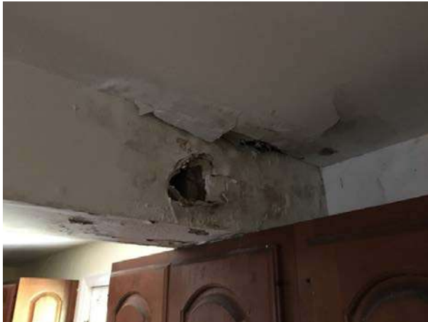
Water damaged drywall in kitchen
