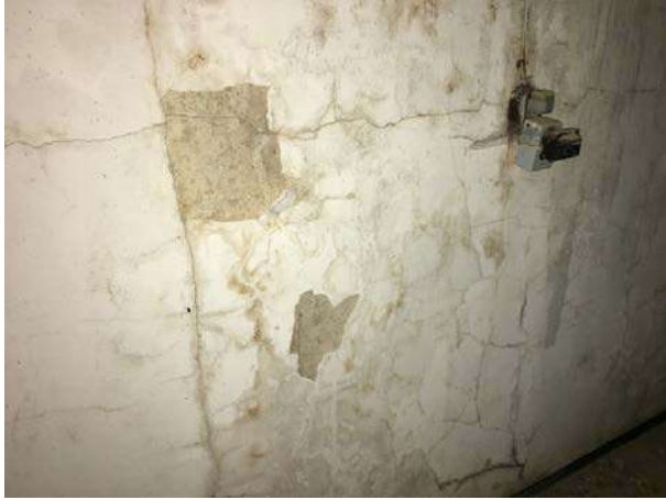
Cracks in the parged walls
