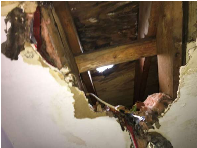
Partial collapse of roof structure.
