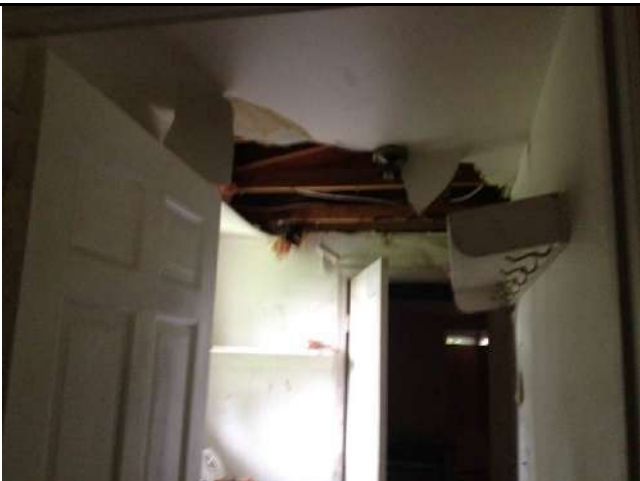
17. View of the ceiling damage from a roof leak in the laundry room/hall.
