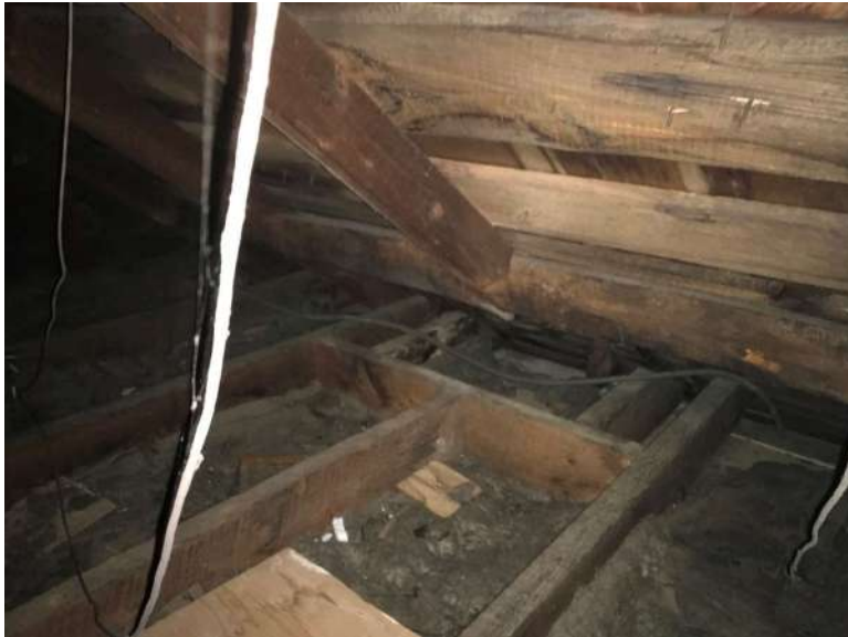
Partial failure of roof framing.
