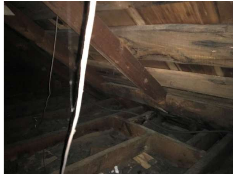
Water infiltration at roof framing. Partial failure of wood framing.
