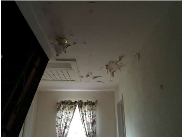
Peeling paint typical throughout building.
