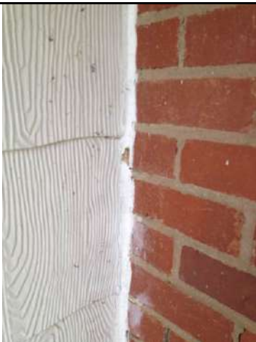
23. View of the tan caulk (ACM) on the chimney of the patio.
