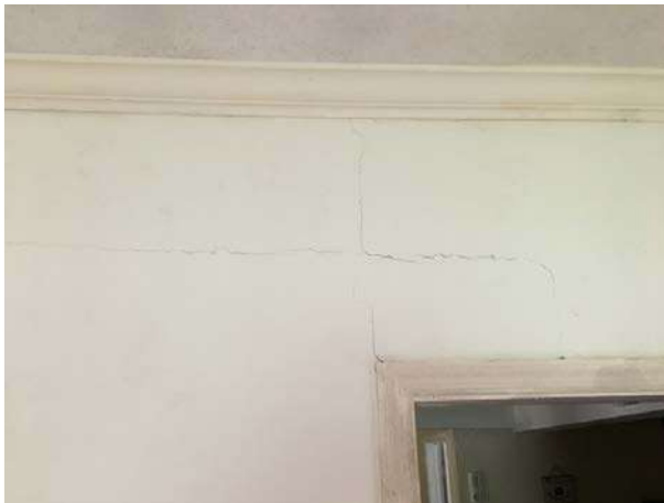
Cracks along a wall
