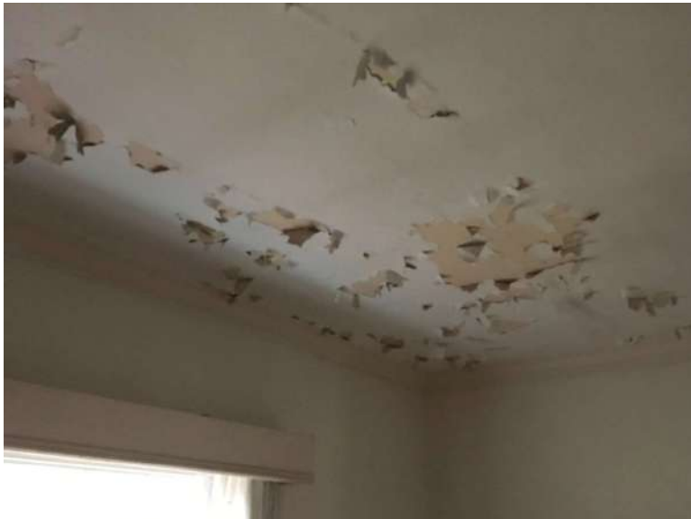
Peeling paint typical throughout building.
