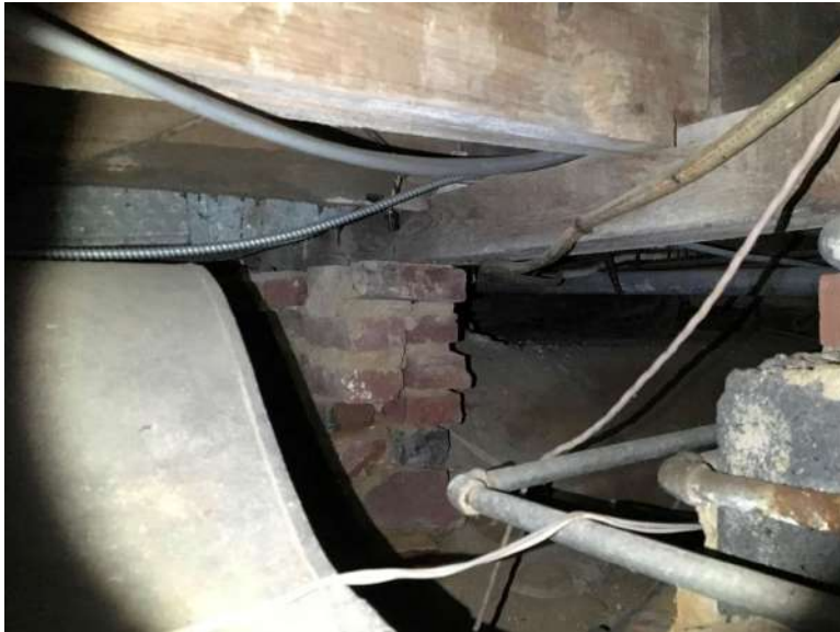
Crawl space under main portion of structure. Significant deterioration of masonry support.
