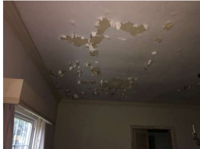
Peeling paint typical throughout building.
