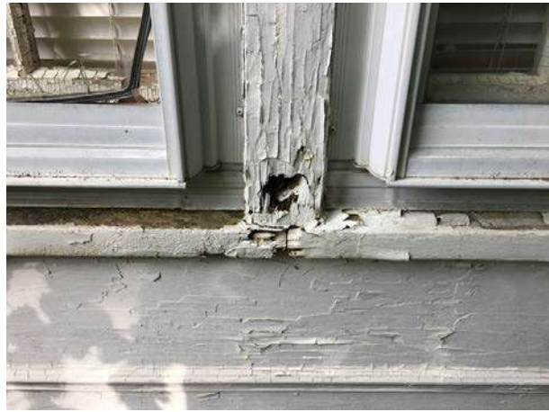
Window frame wood rot
