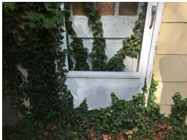
Growth on side door near porch
