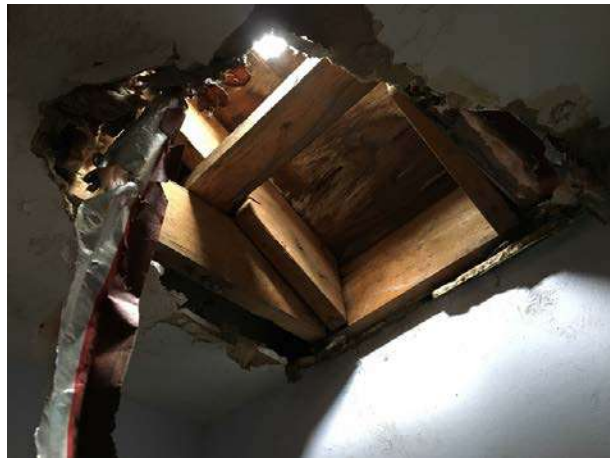
Hole in Roof
