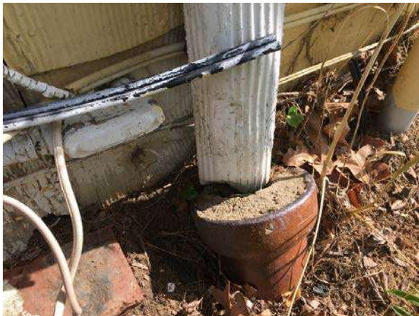
Downspout path blocked
