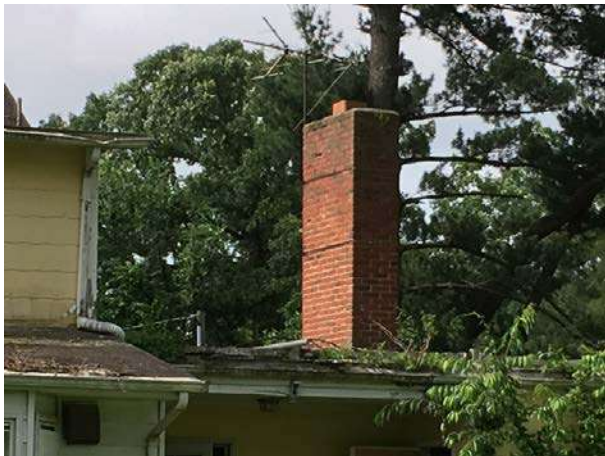
Gutters filled with debris
