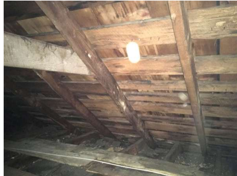
Base of roof rafters appear to have displaced outward. Wood framing appear bowed and twisted.
