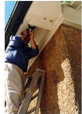
Paint studies may not only help establish the chronology of paints and paint colors used on a building but also may aid in the dating of existing architectural features. Examination of the paint layers on these modillions utilizing a hand-held microscope enabled an investigating team to confirm in the field which modillions were original and which were later replacements. Photo: NPS files.
