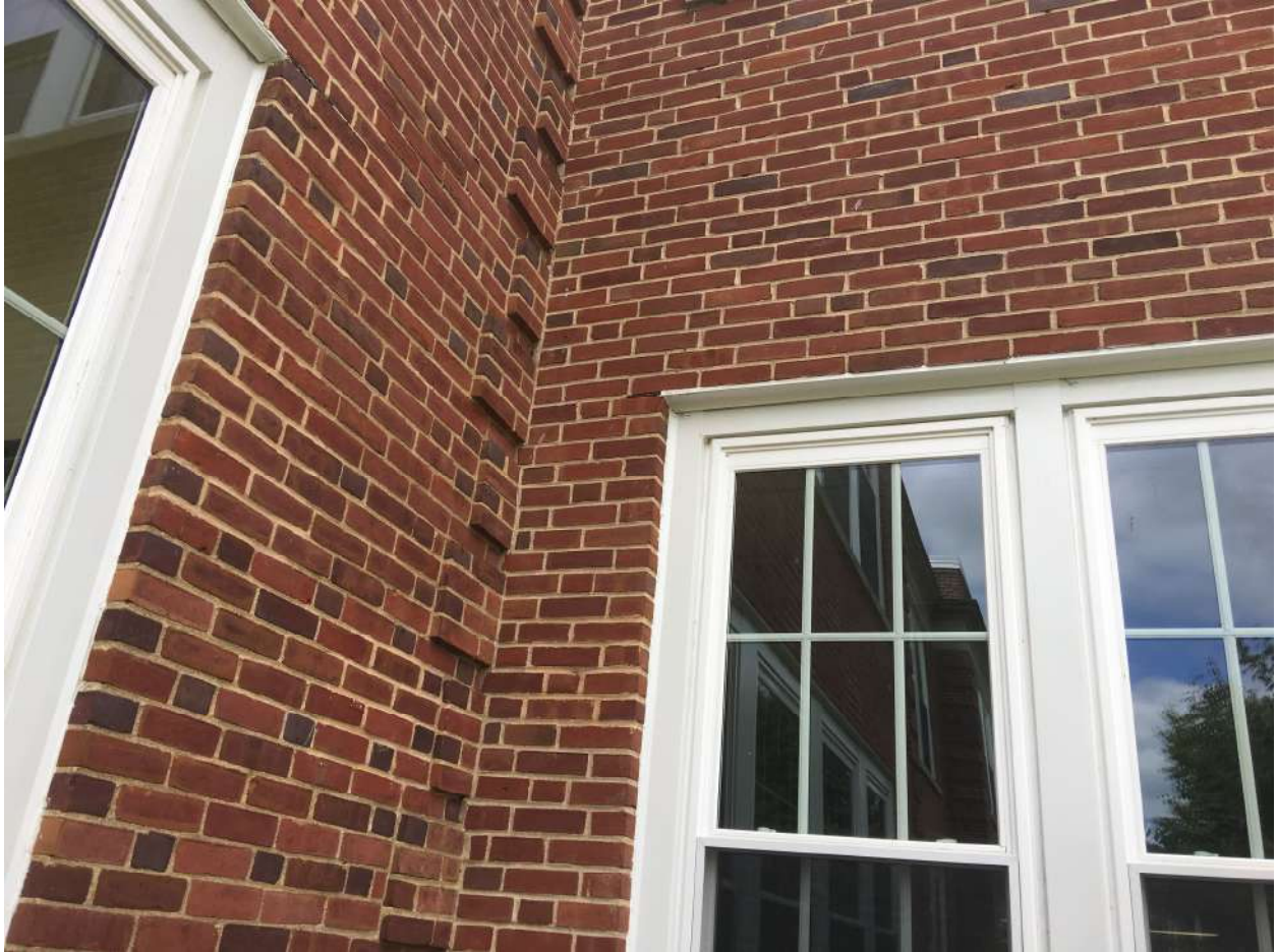
Photo #7: Open mortar joint at corner of window
