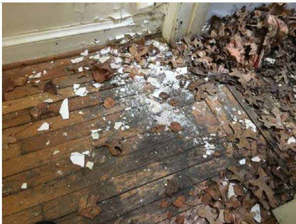
Debris fallen through hole creating possible water damage
