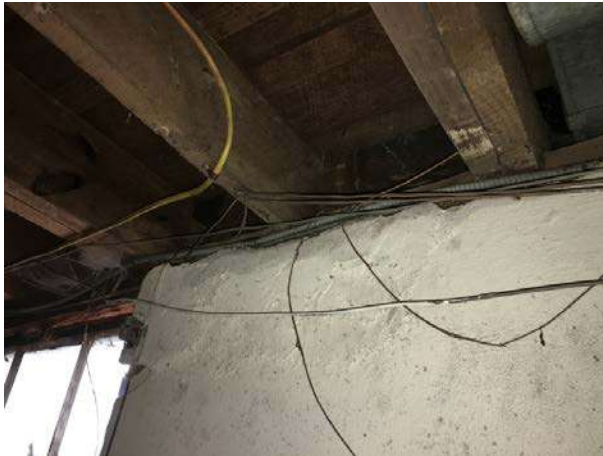
Organic growth penetrating from outside into basement
