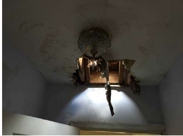
Hole penetrating from roof
