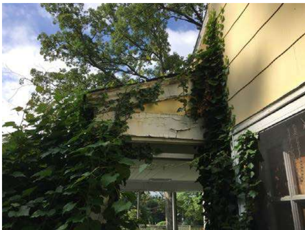
Growth on side porch
