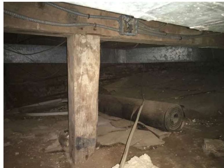
Wood post with crawl space, supporting floor. Wood deterioration.
