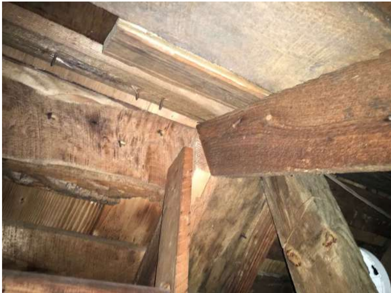
Roof rafters have displaced out of plane along ridge.
