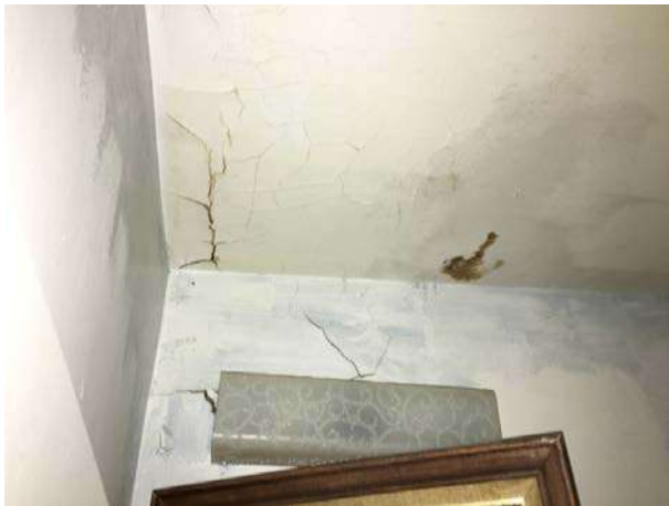
Cracks on a ceiling
