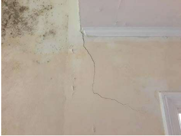
Crack along a wall
