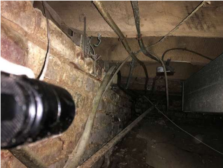
Significant deterioration of masonry foundation.
