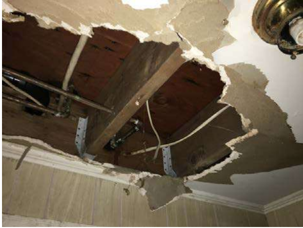
Hole in Laundry Room
