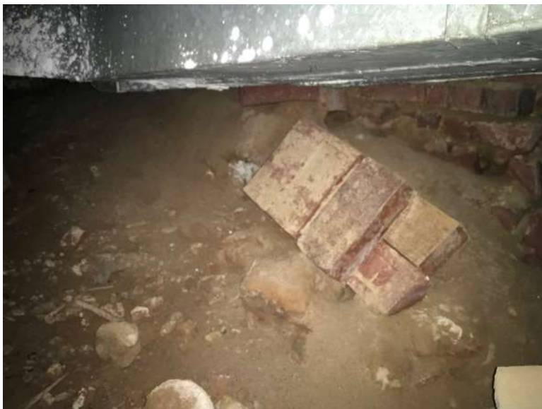
Partial collapse of masonry foundation.
