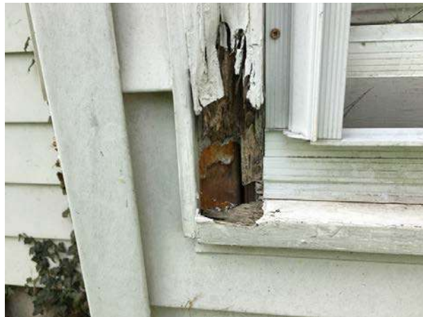
Window frame wood rot
