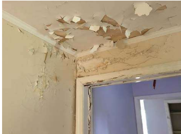
Ceiling paint peeling
