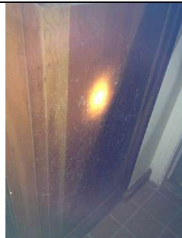
6. View of visible mold on kitchen cabinets.
