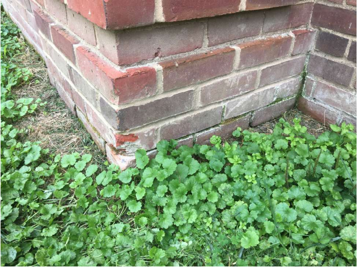
Photo #8: Deteriorated mortar joints at base of exterior wall corner.
