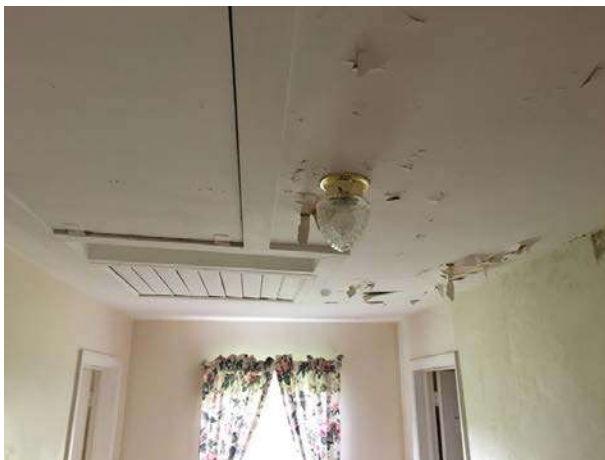
Second floor hallway ceiling sag
