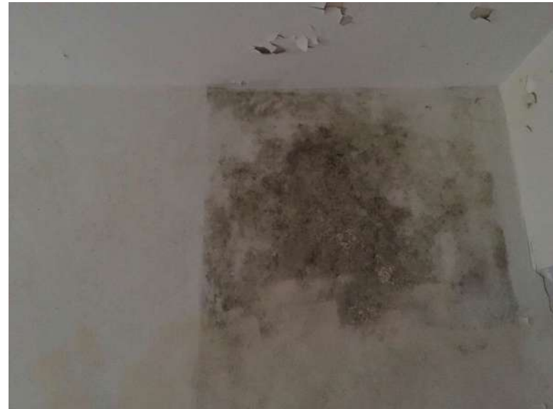
Peeling paint and mold growth.
