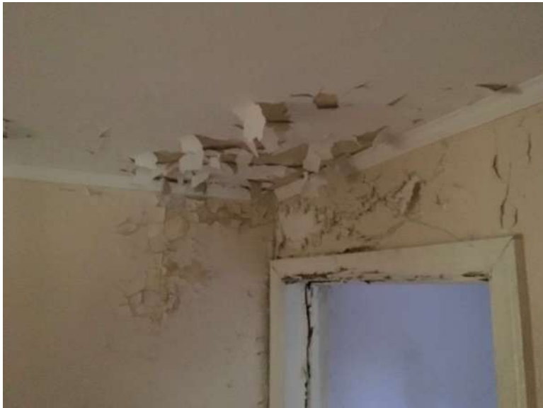
Peeling paint typical throughout building.
