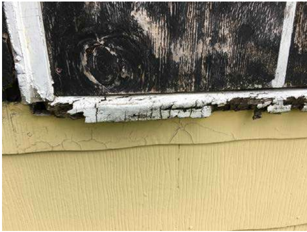
Window frame wood rot
