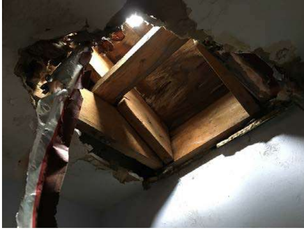
Hole penetrating from roof
