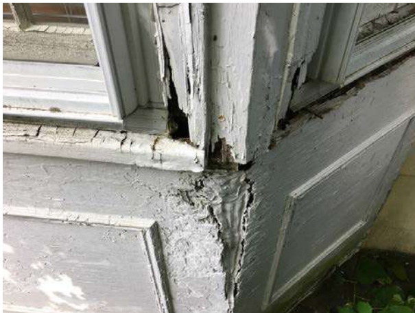
Window frame wood rot
