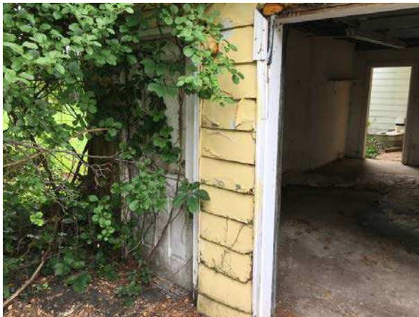
Door Frame damaged
