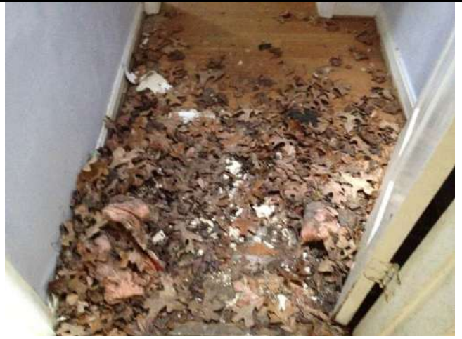
8. View of debris on the floor, partial hole in the floor from the roof leak.
