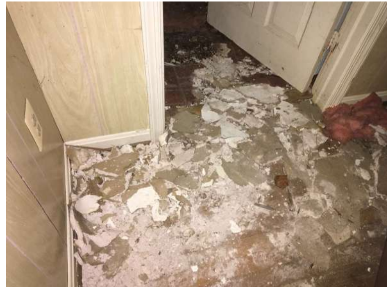
Collapsed ceiling debris on floor.
