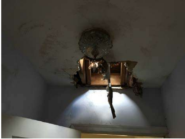
Hole in Roof
