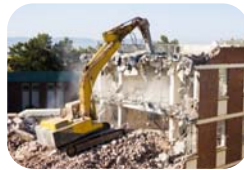
Construction and Demolition Debris
