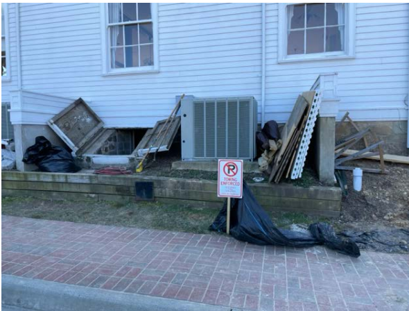
View of Old Town Hall north side HVAC equipment to be removed and relocated. Sanitary sewer is currently behind the timber retaining wall to the left of the visible cleanout.
