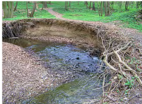
Eroded banks are unstable and susceptible to continued erosion during strong storm events. Erosion can cause stream channels to shift, often impacting private properties and utilities near the stream corridor.
