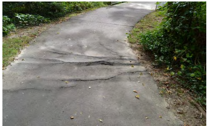
Tree roots upheaving asphalt
