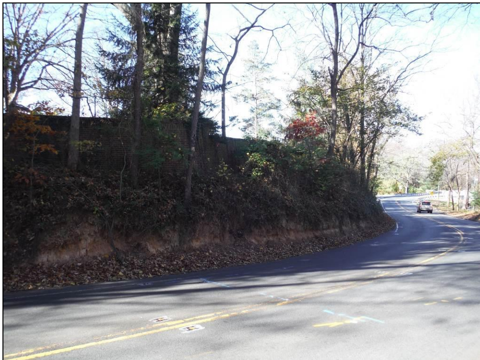
Photo 10: Large Curve Near Northern End of Project Area from East Side of Chain Bridge Road.
